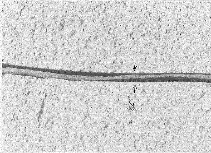
A. Typical Condition of Contraction Joints During Winter Time.
