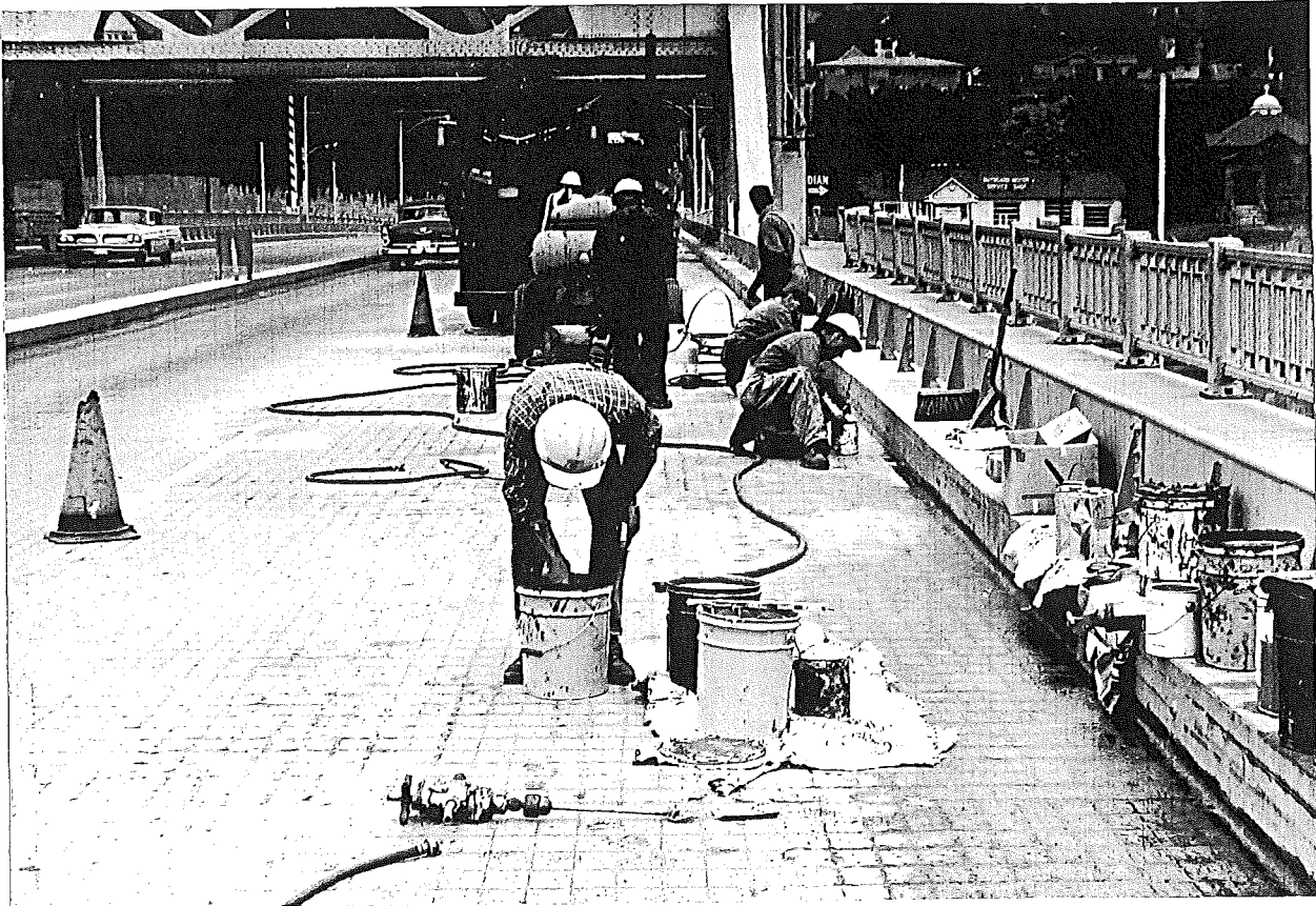
Figure 1. Sandblasting, priming, and mixing operations during joint sealing on the east curb, northbound lanes.
