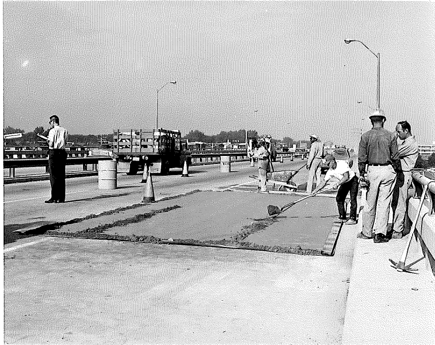
Figure 5. Curing of latex concrete patch in north lane of westbound M 102 (span 8).
