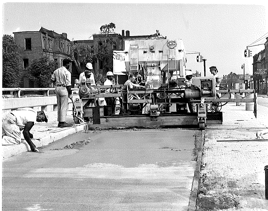
Figure 8. Latex mortar surfacing being placed with vibratory screed and batching and mixing truck. West lane of Brush Street over I 75 (7-16-69).
