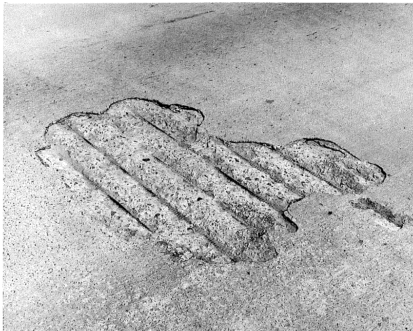
Figure 6. Typical spall development in westbound lane along median adjacent to latex concrete patch (5-1-69).
