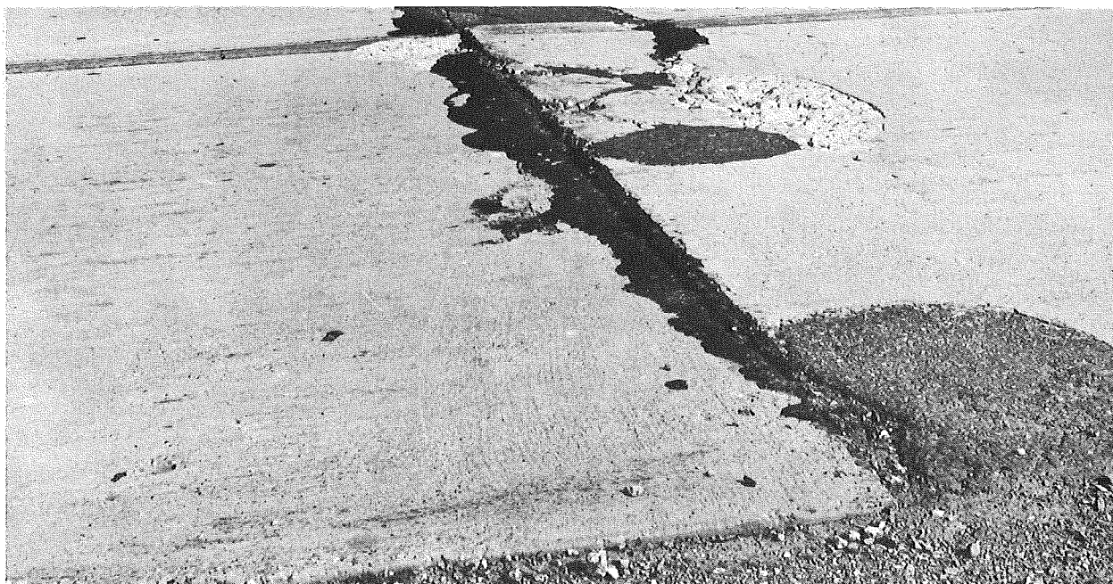
Figure 1. Transverse joint blowup (Sta. 58+36).
