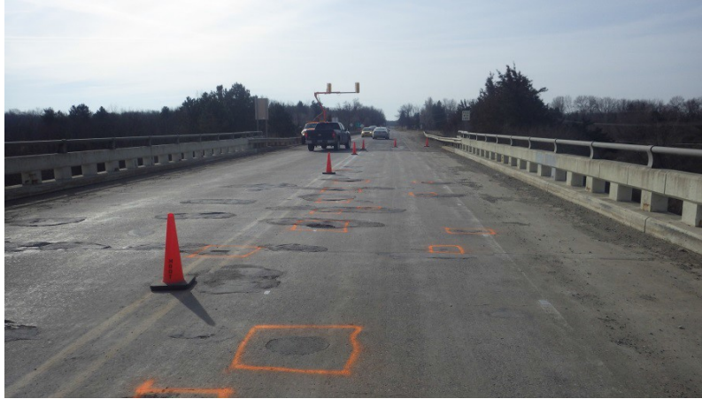
Figure 11: The Lake Nepessing Rd bridge deck was closed to traffic one lane at a time.
