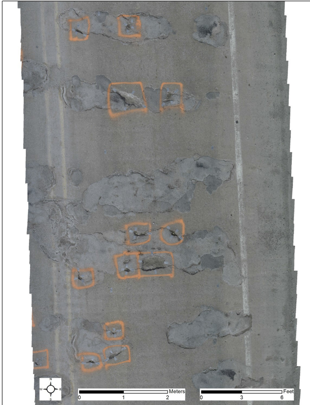
Figure 37: Zoomed in portion of the Orthoimage of northbound Lake Nepessing Rd. bridge deck.
