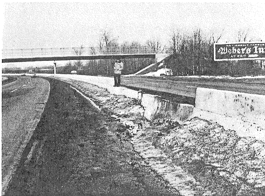
Figure 10. Photo shows where truck climbed snowbank and knocked out concrete glare screen (I-94 near Ypsilanti).
