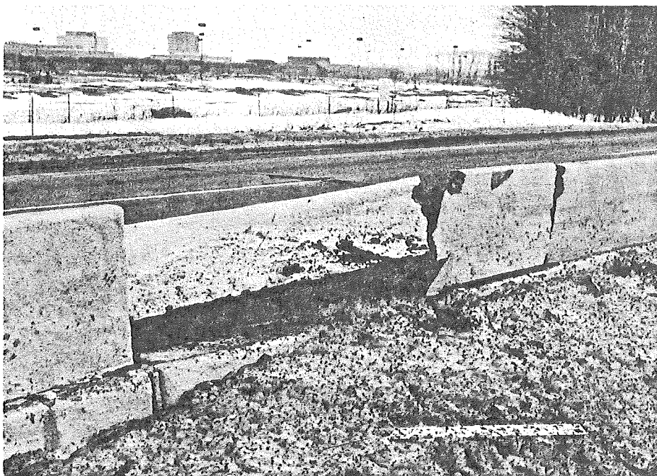
Figure 11. Concrete glare screen probably prevented vehicle from "ramping" over barrier (I-94 in Ann Arbor).
