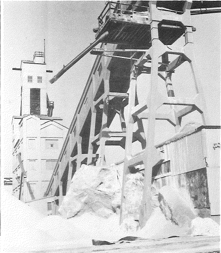
Figure 13. International Salt Co. mine, Detroit. Concrete ramp spray-coated with Gun-Tex 000-SMOOTH in summer of 1961, the old coating having been removed by sandblasting before Gun-Tex application. Concrete pillars supporting ramp have been in contact with salt during entire winter season without apparent effect (photos: 3-1-62).
