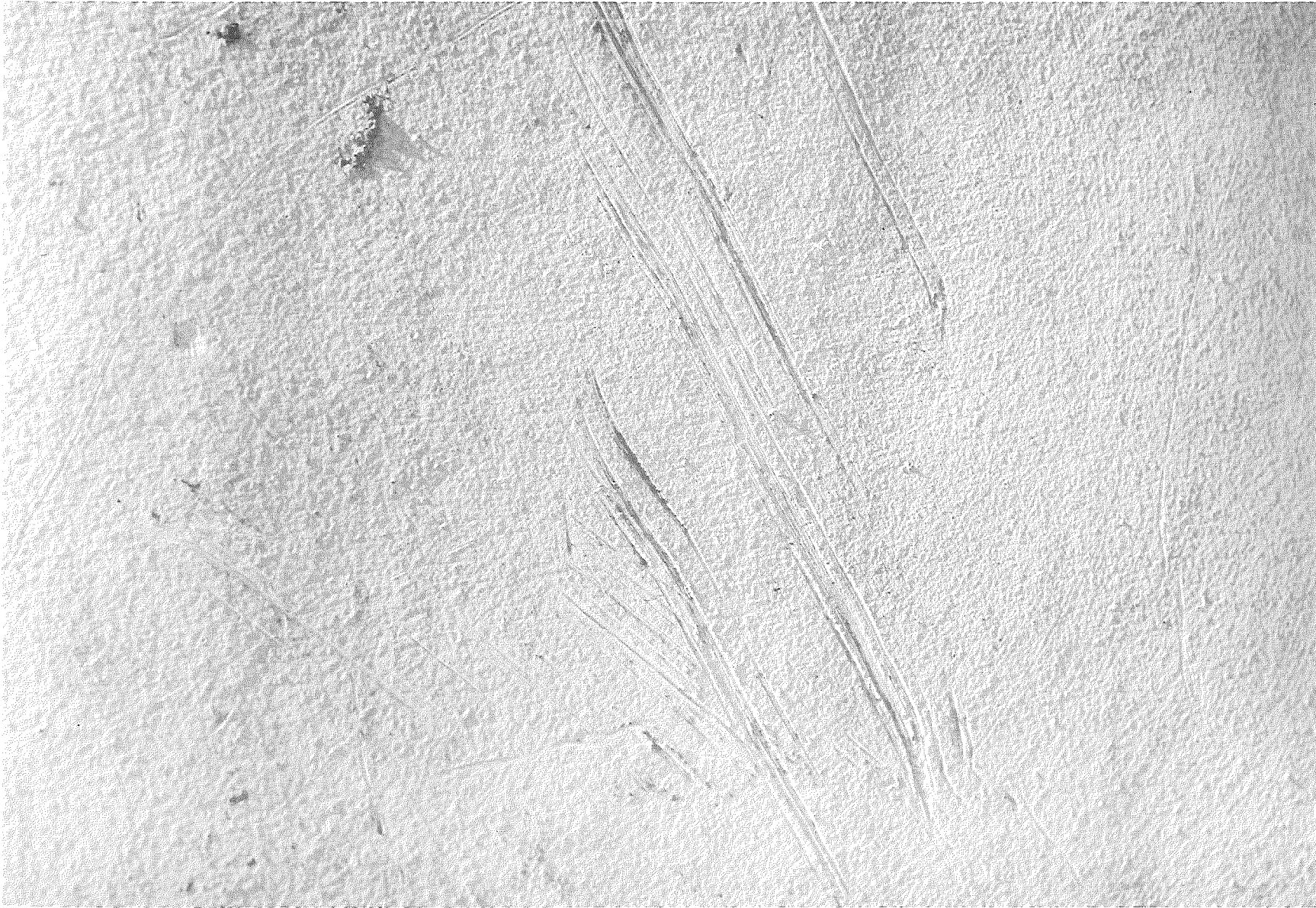
Figure 10. Scuffed area at John K. Orlich funeral home, 17950 Woodward Ave., Detroit. Gun-Tex 000-SMOOTH, white, was applied by spray on June 29, 1960, over badly checked stucco, in one coat at 50 sq ft per gal. Scuffed area shows how material will take this kind of treatment without breaking bond, and indicates depth of coating (photo: 3-1-62).
