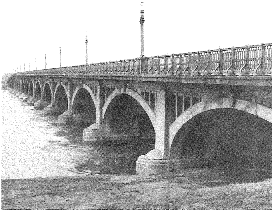
Figure 7. Belle Isle bridge viewed from the island (looking north). Bay on extreme right, which is adjacent to the south abutment, is site of two applications of Armor Speed Finish (photo: 4-9-62).
