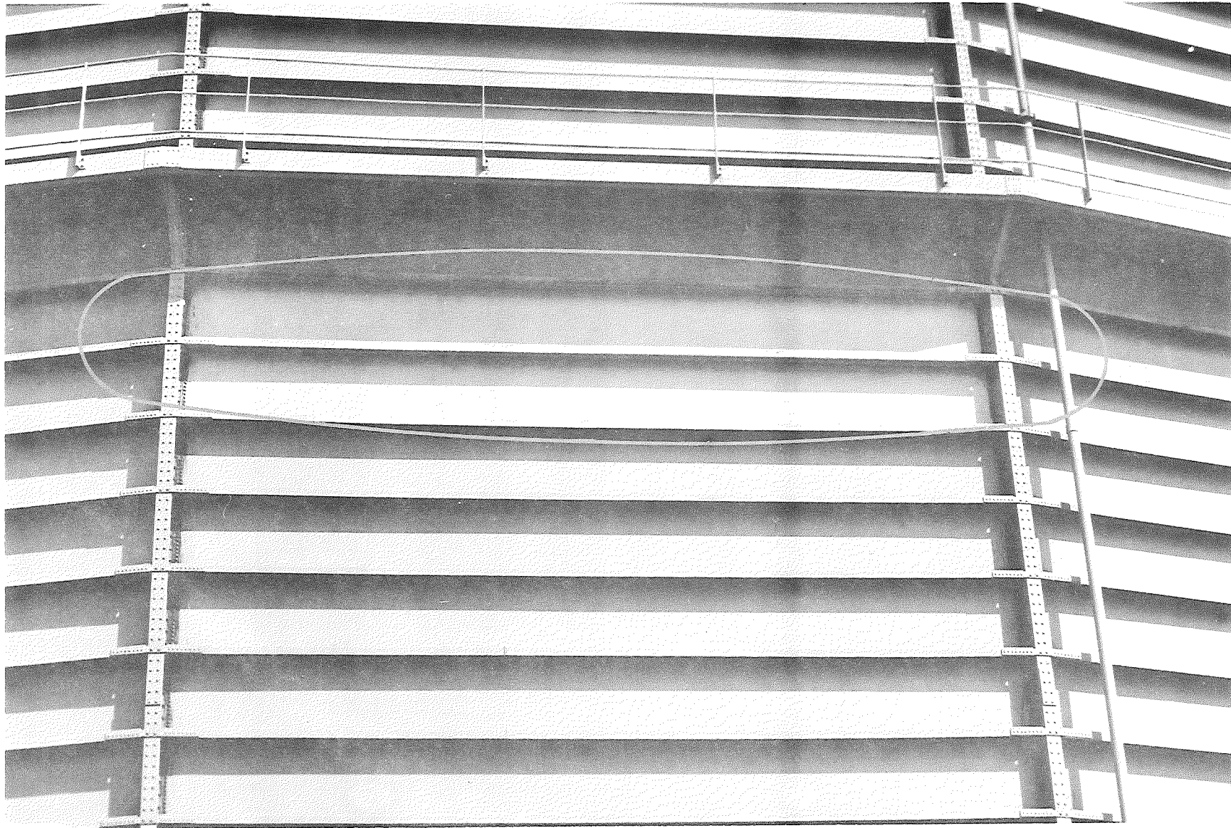
Figure 11. Storage tank of Michigan Consolidated Gas Co. on Lynch Rd. at Detroit City Airport. Two lighter panels (center) were brush coated with Gun-Tex 000-SMOOTH on November 20, 1959, with ambient temperature being below 40 F at time of application. Panels are steel and were sandblasted before coating at 50 sq ft per gal. Coating was in excellent condition at the time of this inspection (photo: 3-1-62).
