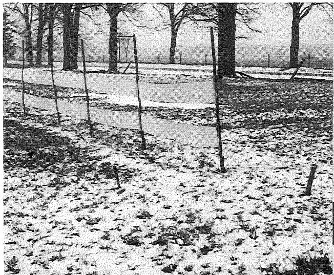
▲ Figure 12. Hillsdale Co., M-49 south of Litchfield. End post braced by tie wire attached to stakes. 2-11-53.
