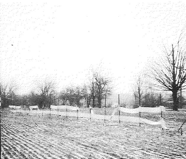
▲ Figure 19. M-99 south of Hillsdale. Damage resulting from improper instal- lation. Paper was not stretched tight. 3-25-53.
