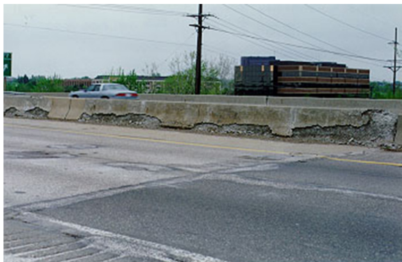
This barrier shows crumbling common in concrete barriers made with blast-furnace slag coarse aggregates—a discontinued practice in Michigan, thanks in part to this study.
