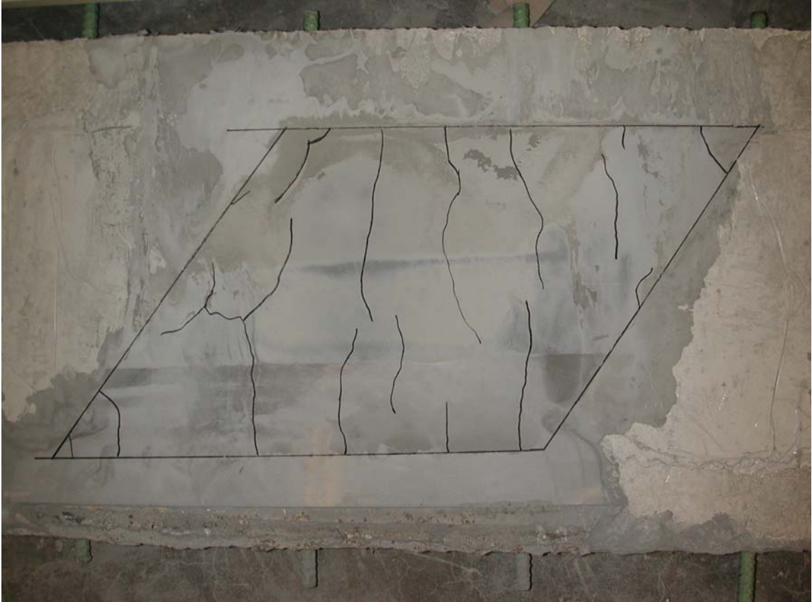
Figure 3.19: Crack pattern in restrained small frame ECC slab (June 30, 2007, the 8 th day)
