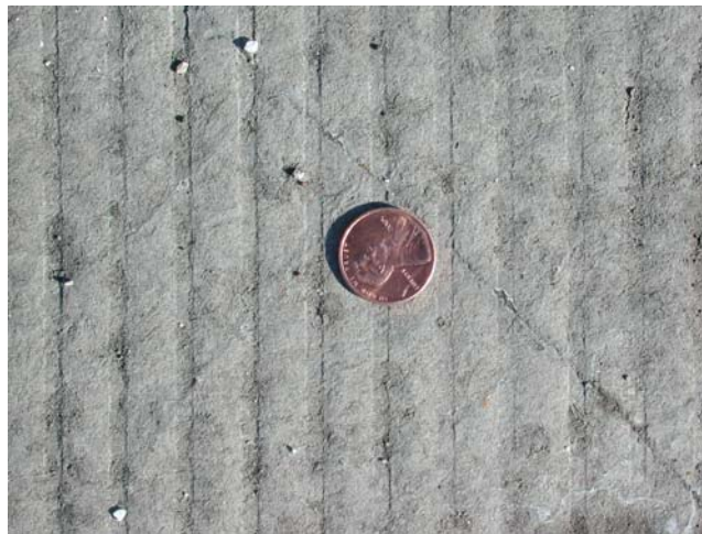
Figure 7.10: Crack width of early age cracks within ECC link slab maintains approximately 0.006" to 0.01" (January 18, 2008)
