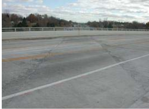
Figure 1.1: ECC link slab on Grove Street bridge over I-94 (S02 of 81063) (completed November 1 st , 2005)
