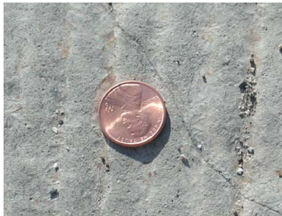
Figure 7.2: Crack width of early age cracks within ECC link slab maintains approximately 0.006” to 0.01” (December 7, 2006)
