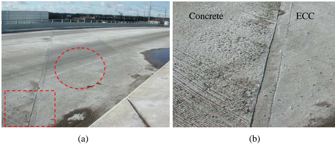
Figure 7.1: (a) 14-month-old ECC link slab on Grove Street Bridge over I-94 and (b) deterioration of adjacent concrete deck enlarged from the area marked with rectangle in (a) (December 7, 2006)
