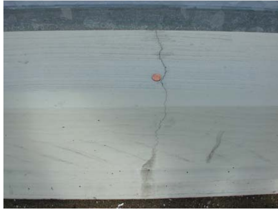
Figure 7.3: Cracking on the concrete railing with crack width approximately 0.02” to 0.04”
