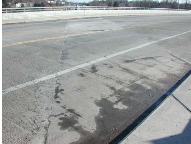
Figure 7.9: 27-month-old ECC link slab on Grove Street Bridge over I-94 (January 18, 2008)
