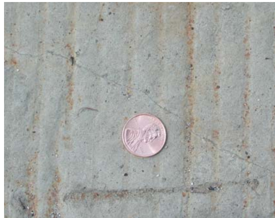
Figure 7.5: Crack width of early age cracks within ECC link slab maintains approximately 0.006" to 0.01" (July 5, 2007)
