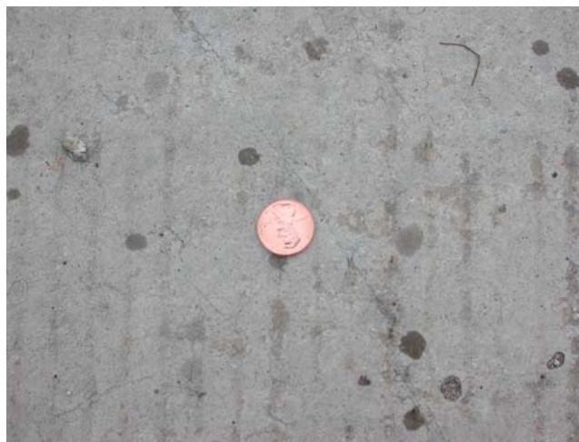
Figure 7.8: Crack width of those early age cracks within ECC link slab maintains approximately 0.006" to 0.01" (October 16, 2007)
