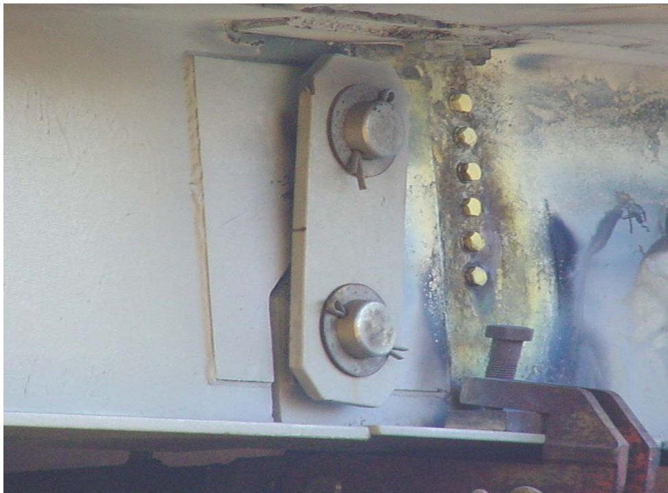
Figure 3.10 Condition of bridge girder after applying strip heat close to pin-hanger detail
