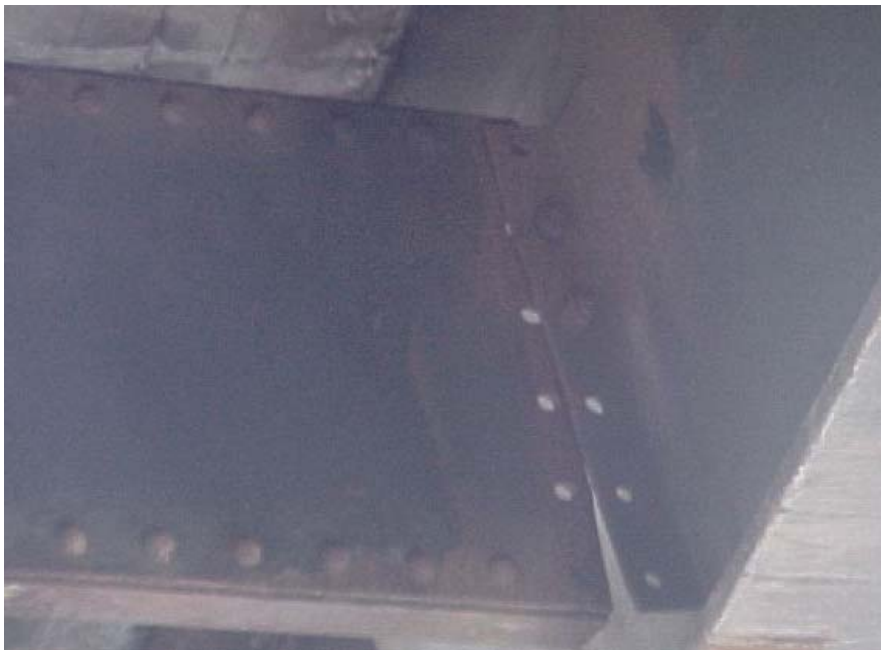
Figure 3.14 Fractured diaphragm-to-beam connection
