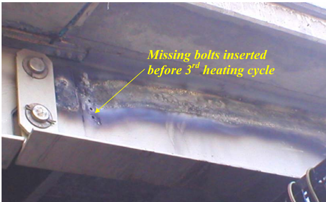
Figure 3.8 Appearance of the Lansing Road bridge girder after two heating cycles
