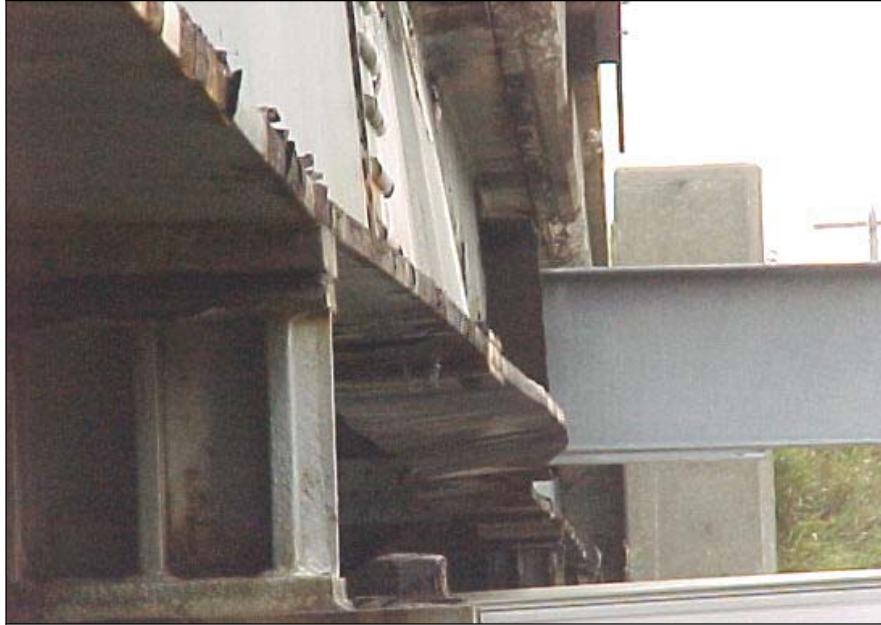
Figure 3.13 Out-of-plane movement of the Elm Road Bridge west fascia beam
