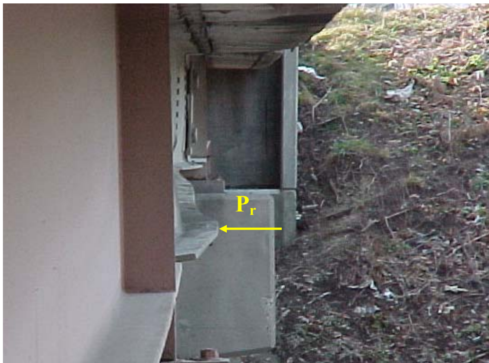
Figure 3.3 Out-of-plane movement of the Lansing Road Bridge west fascia beam
