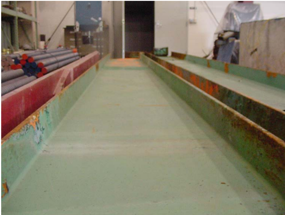
Figure 4.14 Condition of W24 x76 A7 steel beams as received by the MSU researchers
