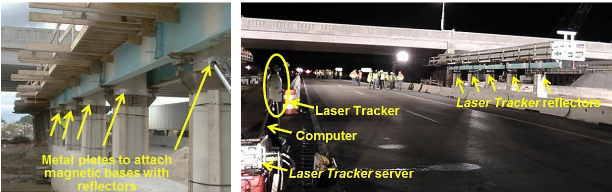
(a) Reflector locations - metal plates to attach magnetic bases with reflectors (b) Laser Tracker, controller, and the computer at the site
