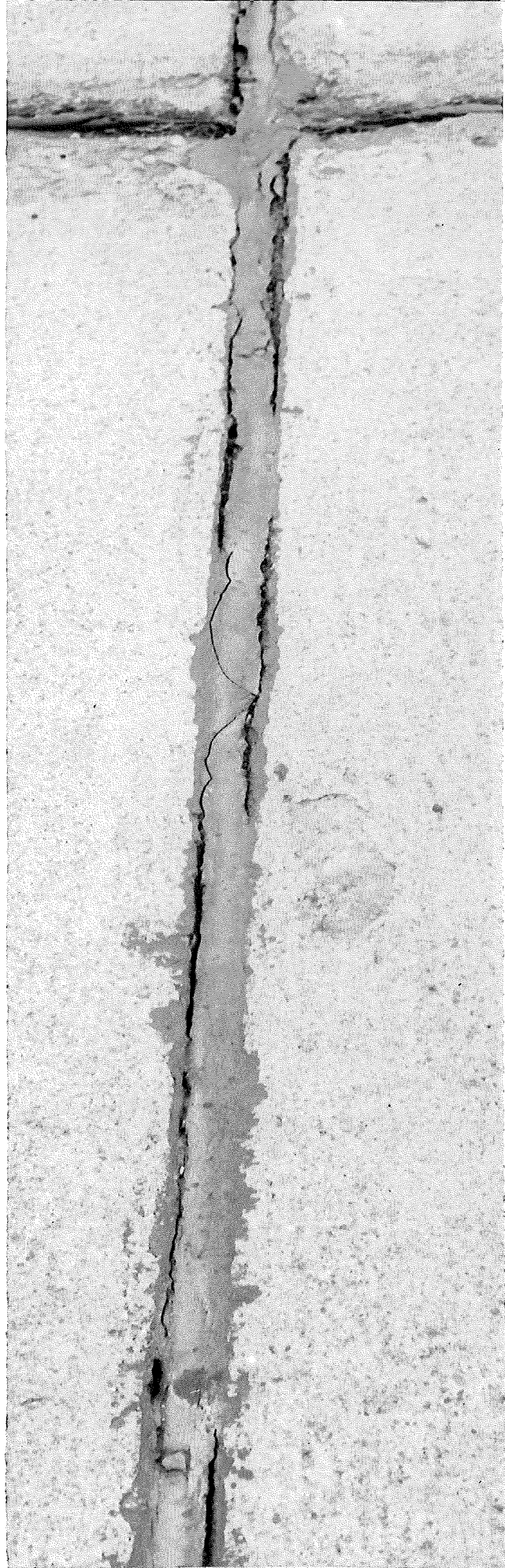
Material B, Station 160+90 Failures in cohesion.
