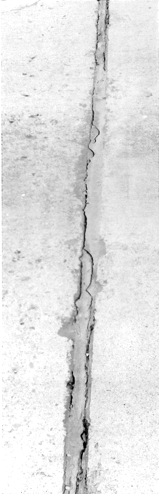
Material A, Station 177+80 Failures in cohesion.
