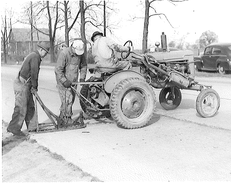
Figure 2. Plow used for cleaning out old joint seal in preparation for resealing of expansion joints.
