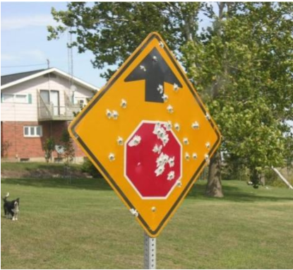
Signs with extensive gunshot holes should be replaced.
