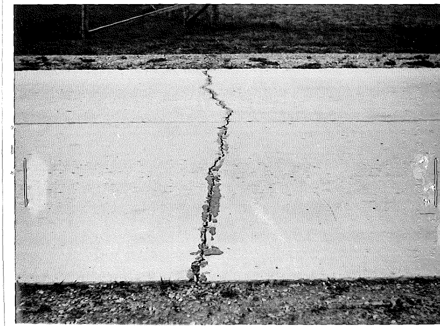
Figure 5. Typical condition of cracks when only one or two appear per 300 foot slab, approximately 1/8 inch opening.
