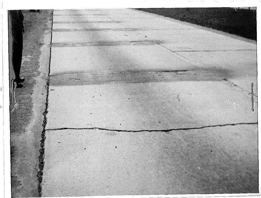
Figure 8. Badly cracked and faulted area on Queens Highway, East of Hamilton, Ontario, looking east. This pavement carries west bound traffic to Hamilton. Faulting as much as 1" was observed in some instances.
