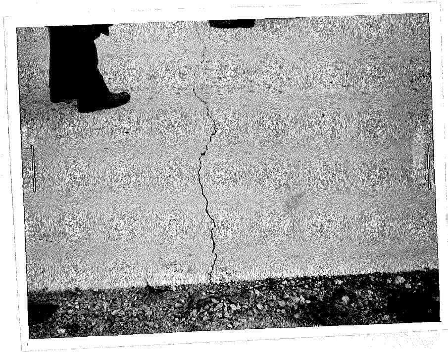
Figure 4. Typical condition of cracks in most slab lengths of 300 feet. Approximate width 1/8 inch.
