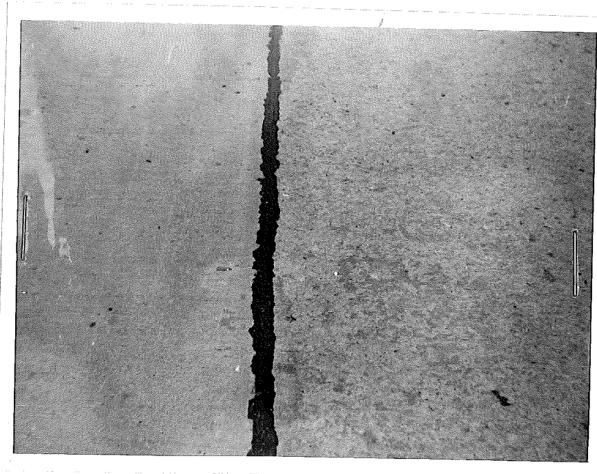
B. Close view showing general condition of adjacent sealed and unsealed surfaces.
