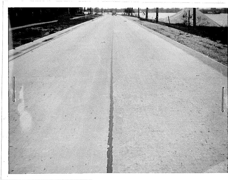
A. General view looking south showing scaling of the west lane constructed with normal Portland Cement. East lane was constructed with Vinsol resin cement.
