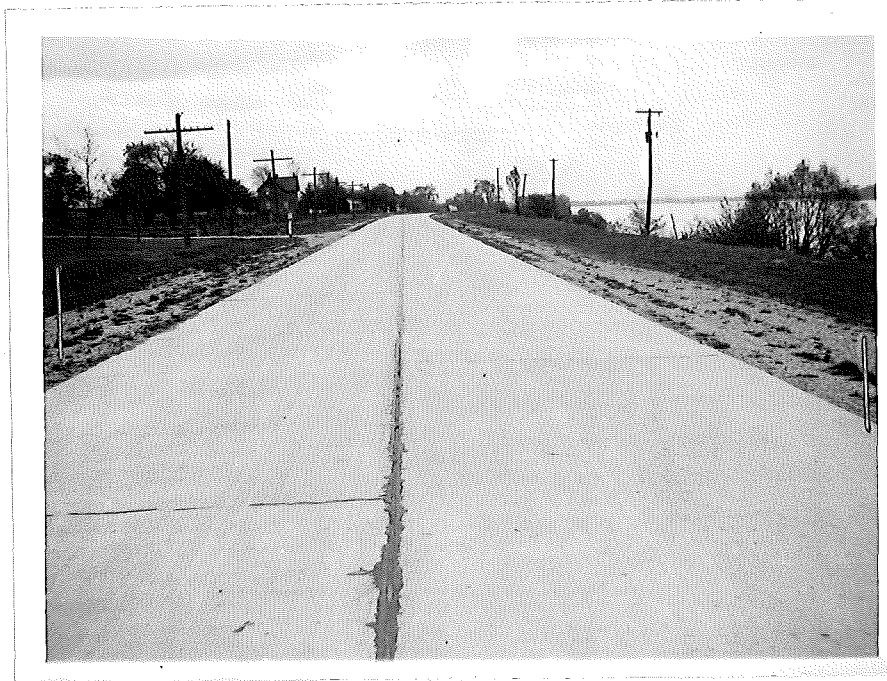
B. Same project looking south showing relative cracks in east and west lane. West lane 2 to 3 cracks per 300 foot slab East lane 5 to 6 cracks per 300 foot slab
