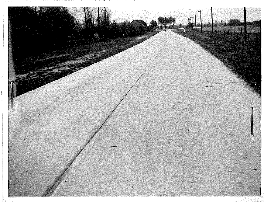
Figure 7. Typical condition of pavement ten years old with 8 to 10 cracks per 300 foot slab length. Cracks have not been filled which would have made them quite discernable in photograph.
