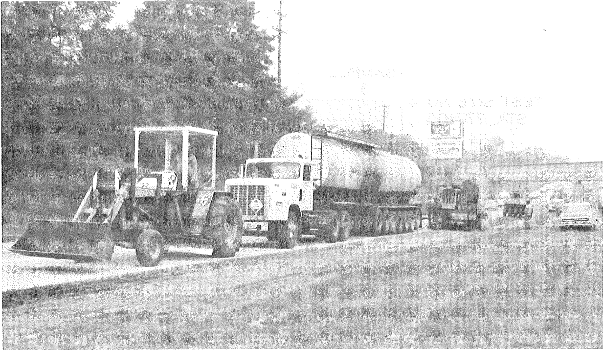
Stabilization of median shoulders along I 96BL in Muskegon County. Operations include asphalt tanker (pulled by tractor), single-pass stabilizer adding and mixing foamed asphalt, and pneumatic roller.
