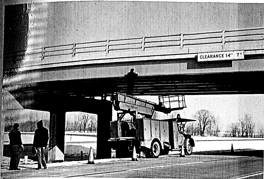
Figure 1. Condition of bridge coatings inspected using Office of Maintenance Strato-Bucket on M 71 over M 78.
