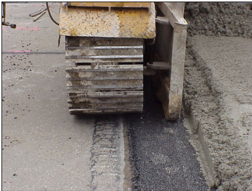
Figure A9. MDOT Report # R-1465, Figure 5, Paver Track Running on Asphalt Separator Layer
