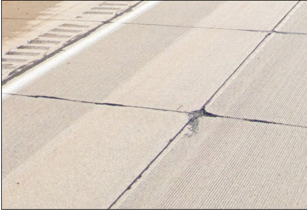
Figure A16. Minor Corner Cracking in Section 5 on Northbound I-75 (Google Maps, Image Capture: September 2019)
