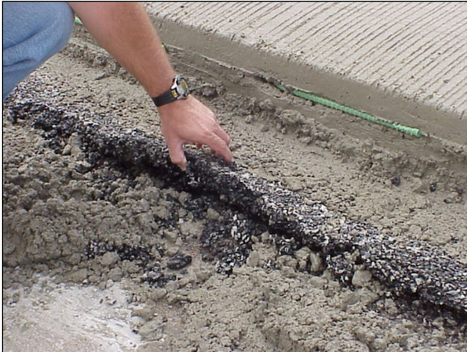
Figure A10. MDOT Report # R-1465, Figure 7, Loose Asphalt Separator Layer. Note Embedded Lane Tie That Can Not Be Straightened for The Adjacent Lane
