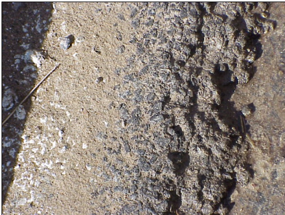
Figure A11. MDOT Report # R-1465, Figure 9, Voids in The Separator Layer Are Plugged with Construction Debris
