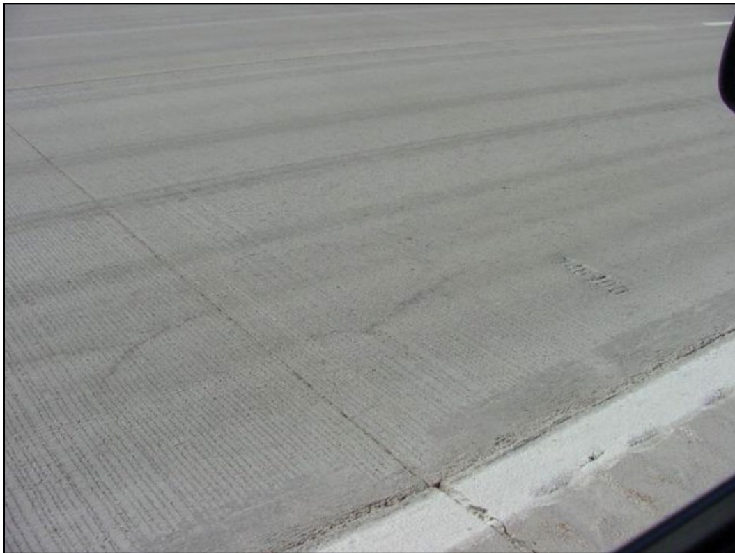
Figure A19. MDOT Report # RC-1574, Figure A11, Start of Longitudinal Cracking at Joints in Section 3 Within Year 1 (October 2004)
