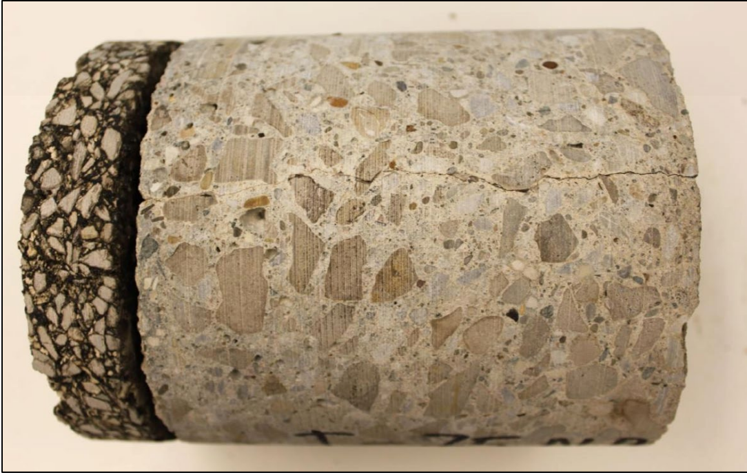
Figure A20. MDOT Report # RC-1574, Figure A12, Top-Down Longitudinal Cracking Starting at Transverse Joint Station 709+08 (Section 3)
