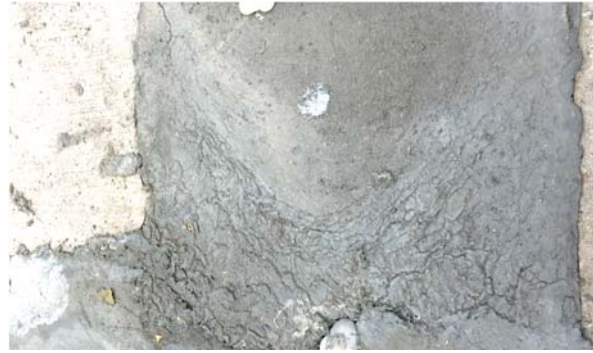
(b) Shrinkage cracks on the surface
