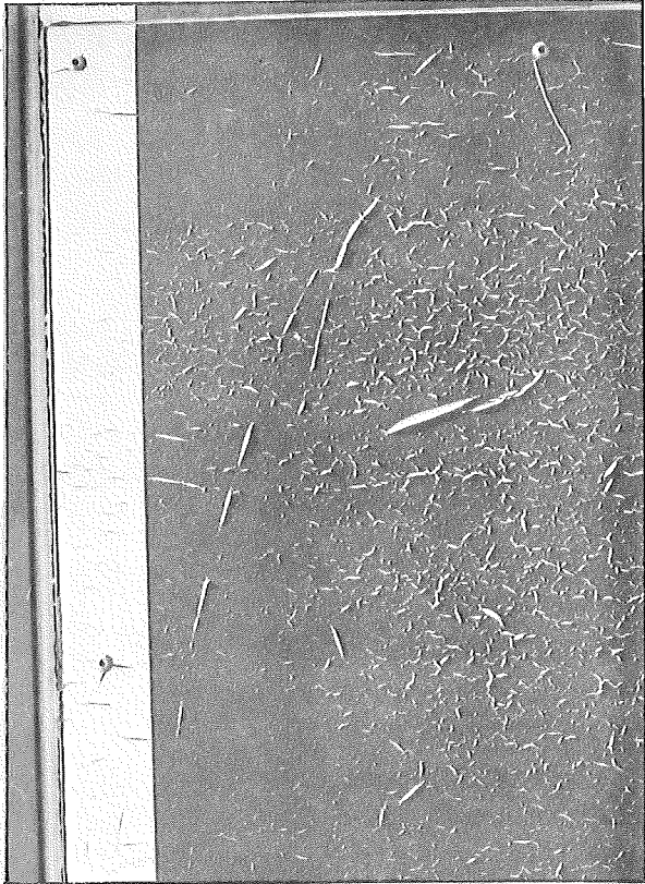
Figure 7. Daytime view of 3M sign (1978) showing severe peeling and crazing.
