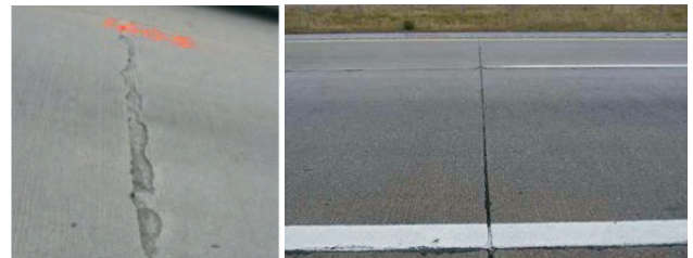
Sections of US-23 test road: (left) Typical transverse mid-panel crack spalling in Section B (blast-furnace slag aggregate) in 2006. (right) A typical transverse joint found in Sections A through E in 2016. There was no sign of deterioration at the joints.
