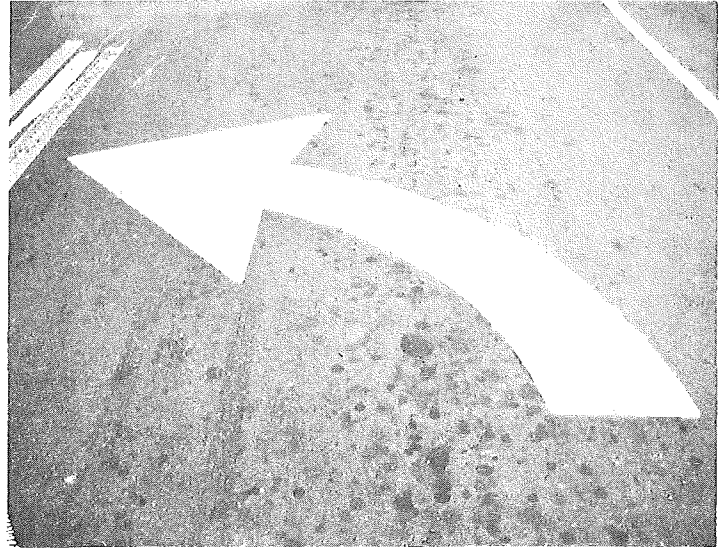
Arrow # 10 Location I 10/27/70 Holland-Suco Left Turn Arrow
