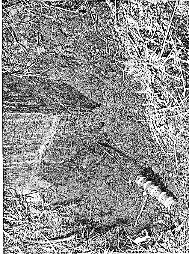
Figure 2. Creosote treated post allows only minor penetration of probe below ground line signifying sound wood. Post is 18 years old on southbound US 27 near north Clinton Co. line.
