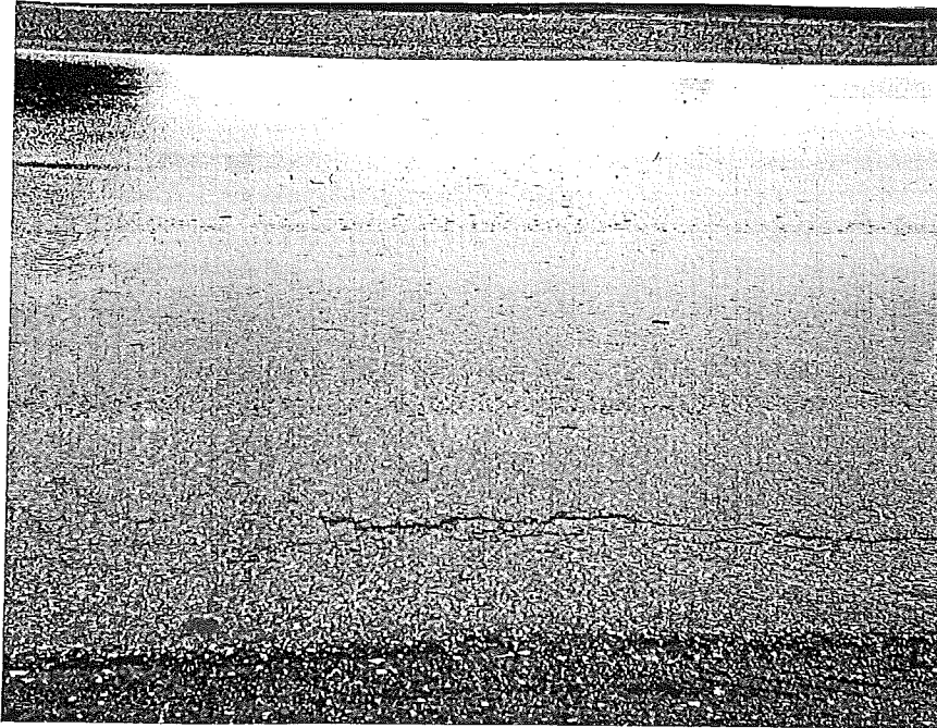
A. Typical condition of surface. Slight pitting (raining).
