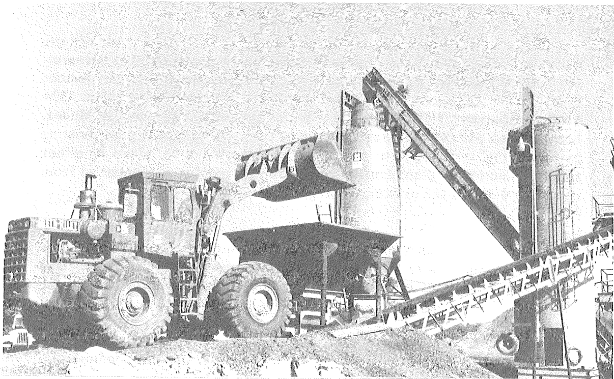
Figure 2. Method of feeding reclaimed material to the weigh hopper.
