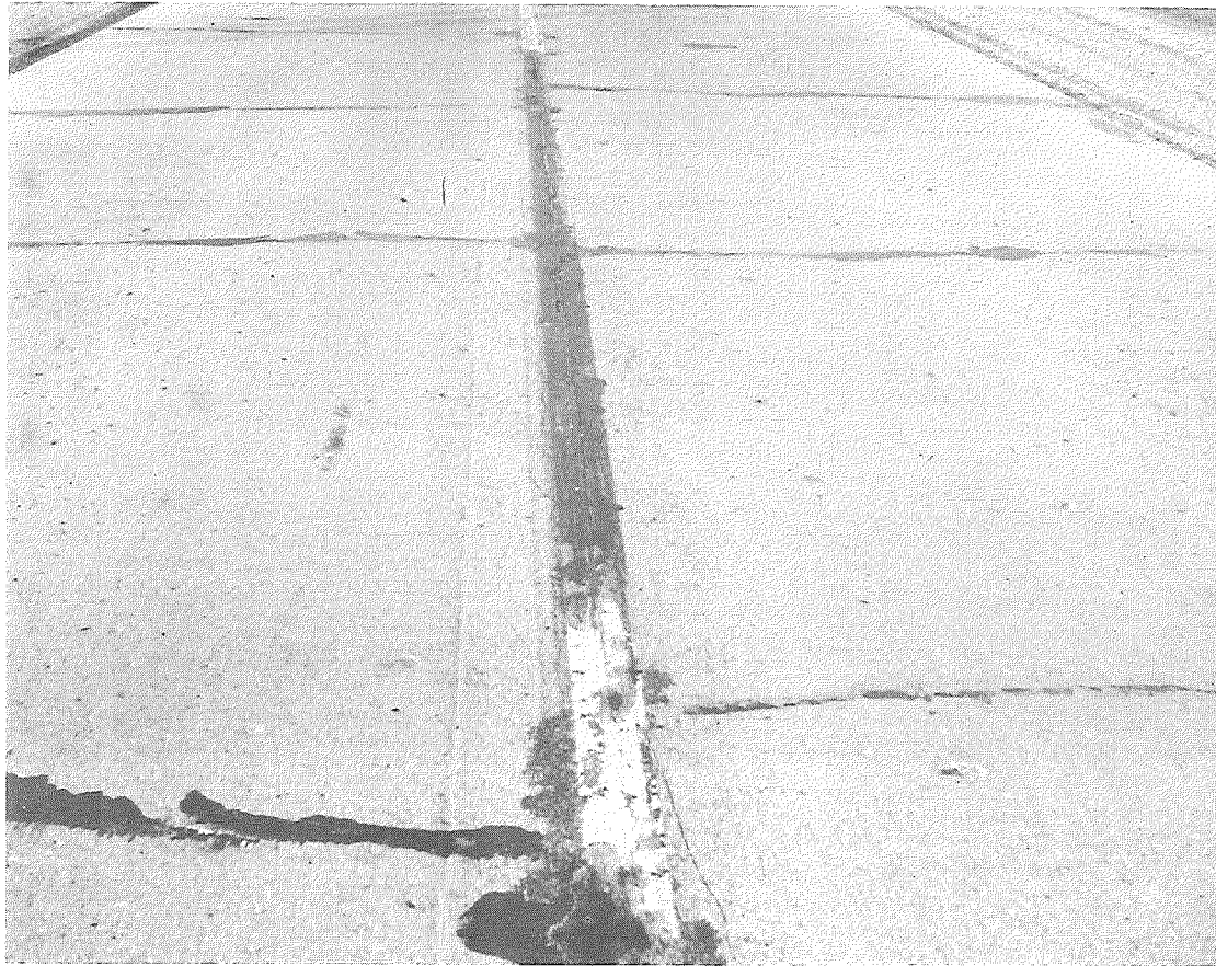
▲ Station 487 looking north. Popouts and frequent transverse cracks were encountered on even the best sections of Contract 5.
