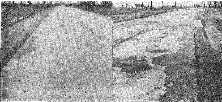
▲ Station 249 looking South. Edge disintegration without presence of serious cracking was frequently found in Contract 4. Built in 1934, this section's wire mesh reinforcement seemed to have effectively controlled cracking for more than 20 years (POB at top of Figure).
