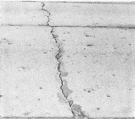
▲ Station 49+78. Typical of cracks in non-reinforced concrete sections.
