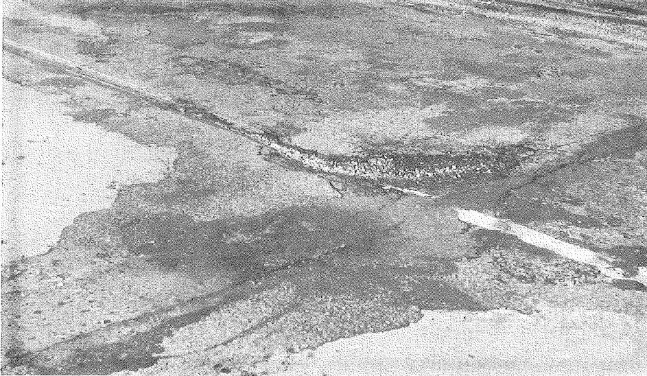
▲ Station 288. In 1955, a blowup developed at a tar-patched joint on this badly disintegrated and multipatched slab.
