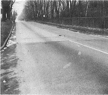
▲ Station -20+17 looking north. The widened urban section of US 27, built by part-width construction, has a generally smooth-riding surface. Slight faulting occurred at the transverse joint in foreground.
