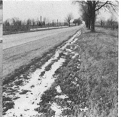
▲ Station 48, looking north. Drainage was blocked along much of the route, with tire ruts crossing shoulders and ditches.
