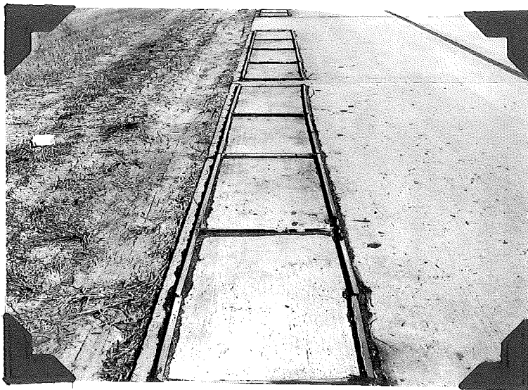
Figure 2B. Rock Salt panel of test area No. 4 in foreground after 30 cycles. Concrete 7 years old. No scale.
