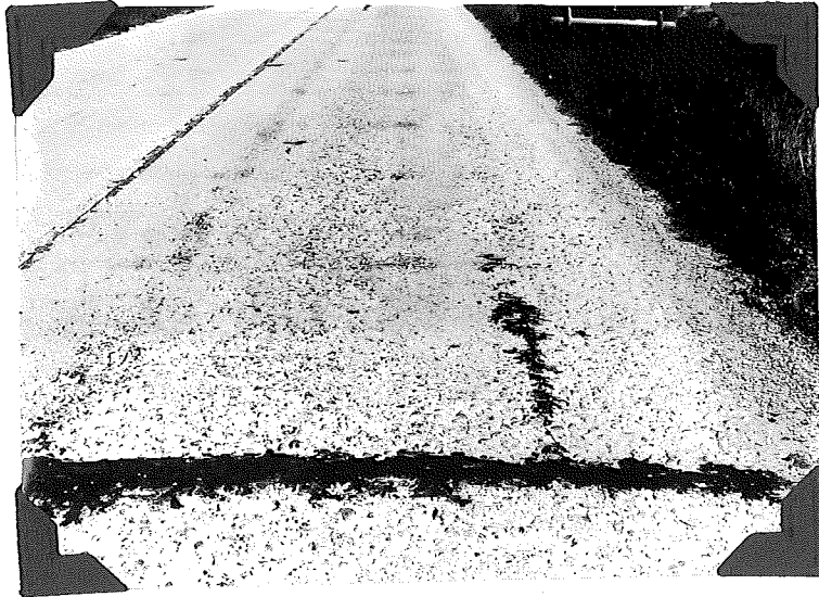
Figure 6. Photograph showing the effect of chloride salts on concrete containing inferior aggregates.
