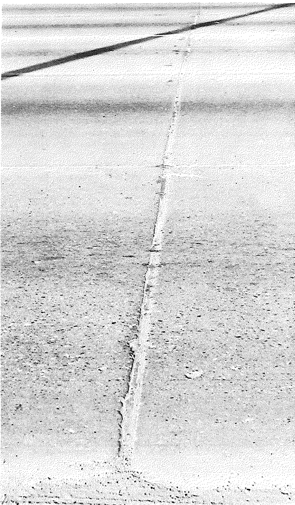
Figure 6. Typical sound contraction joint in 5-in. capping and adjacent widening (foreground), after 7 years. (Feb. 1960). 4+41 - Method 1.
