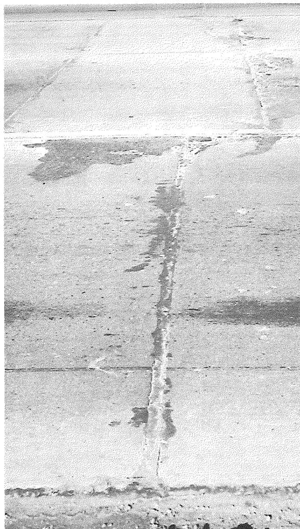
Figure 7. Joint failure in 5-1/2-in. capping, resulting in patching of center lanes (Feb. 1960). 7+35 - Method 1.
