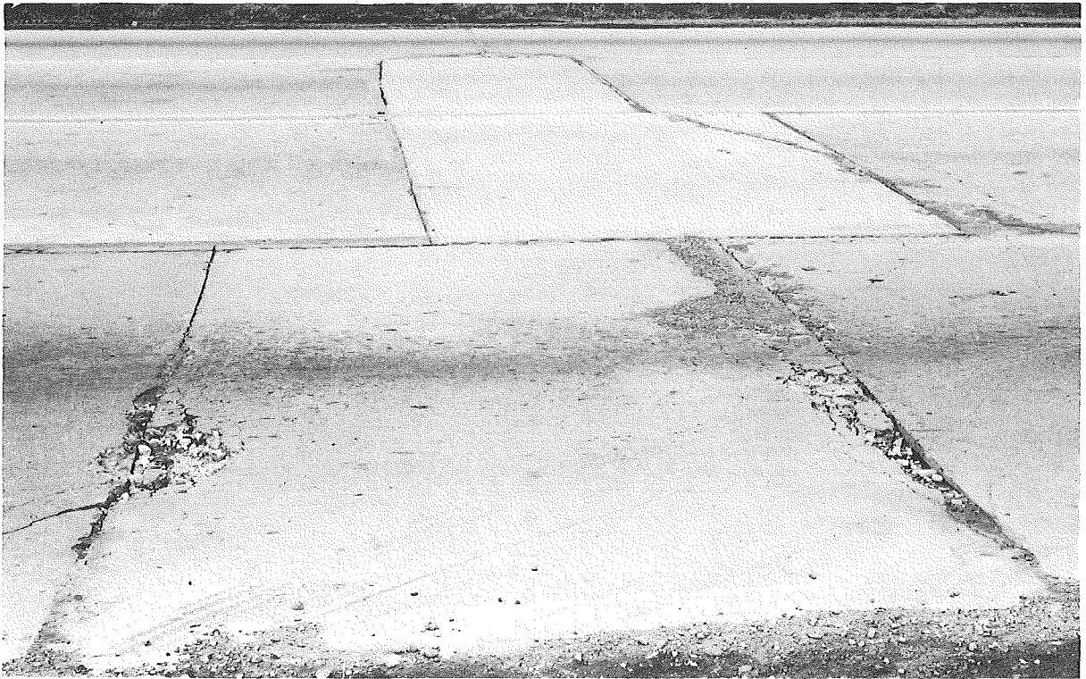
Figure 20. Repaired area at contraction joint in 6-in. capping (center lanes), with similar repair in foreground widening lanes; note concrete deterioration in widening patch (Dec. 1959). 301+97 - Method 4.
