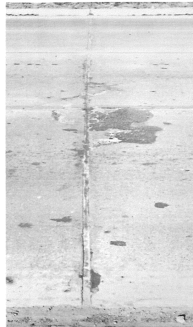
Figure 8. Minor joint deterioration in 5-1/2-in. capping and adjacent widening (Feb. 1960). 28+33 - Method 1.
