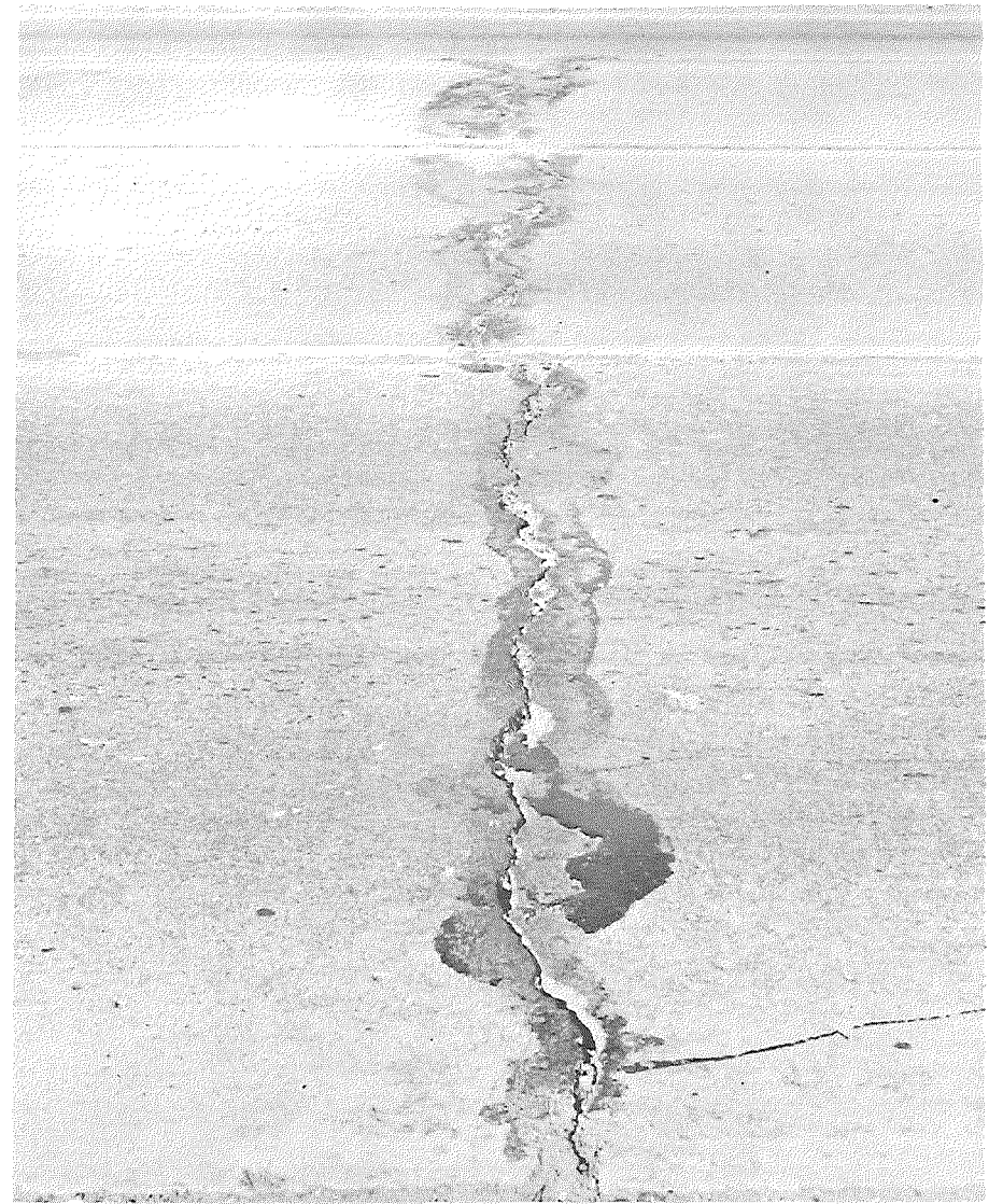
Figure 15. Crack in 6-1/2-in. capping continued in foreground widening lane, after 7 years (Feb. 1960). 350+48 - Method 2.
