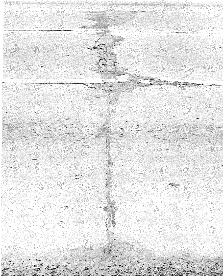
Figure 14. Contraction joint deterioration in 6-1/2-in. capping (center lanes) after 7 years (Dec. 1959). 353+67 - Method 2.
