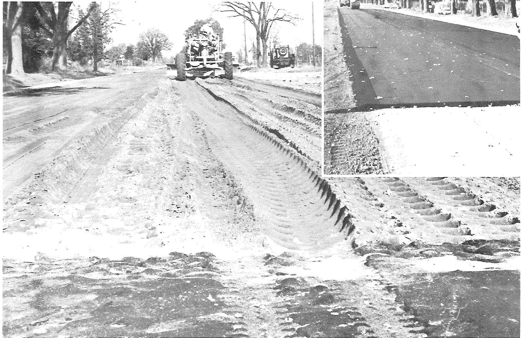
Figure 6. Asphalt-stabilized bank run gravel (right), and attempted compaction of bank run sand (left).
