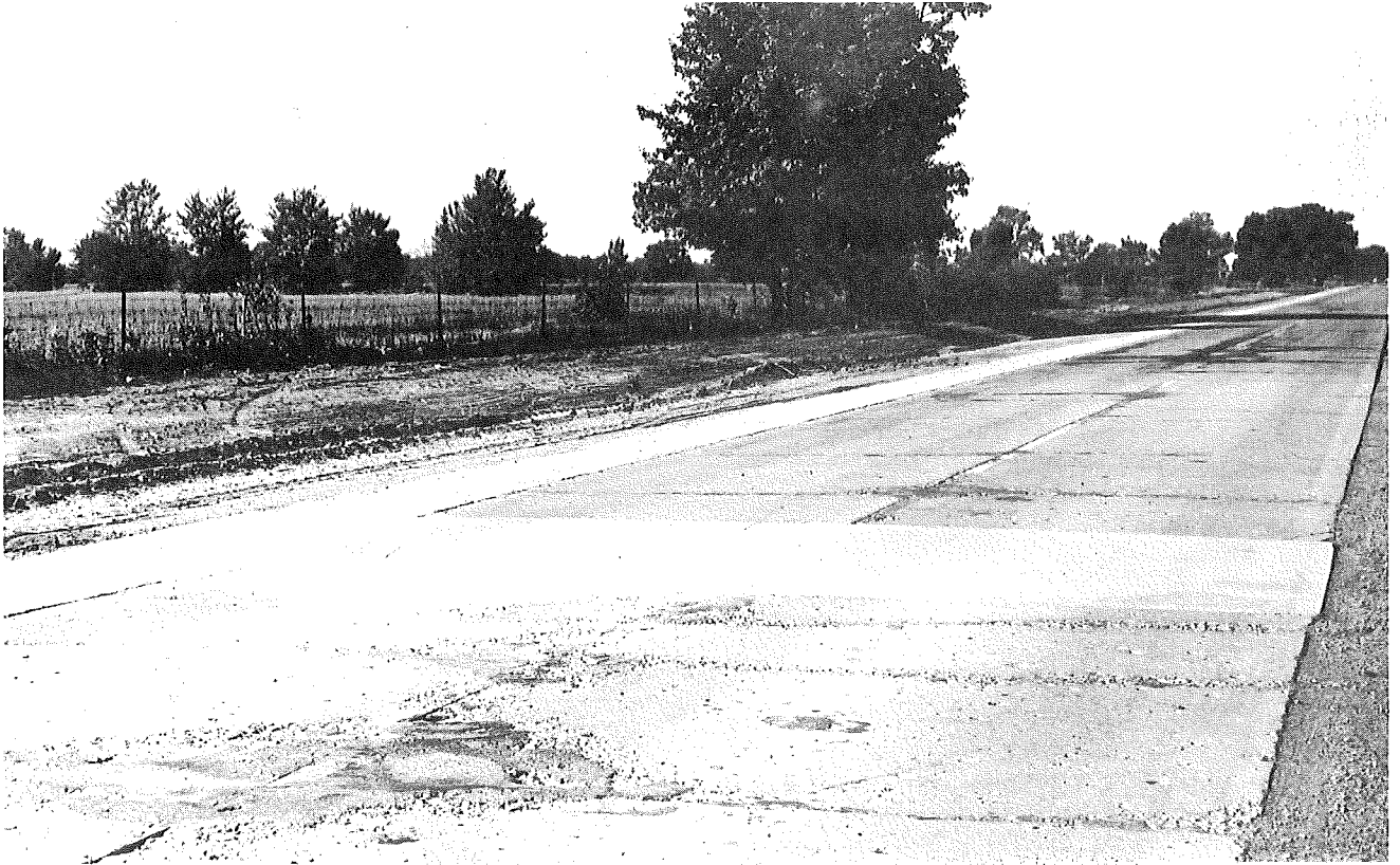
Figure 3. Original rigid pavement. Note transverse patch replacing blowup.
