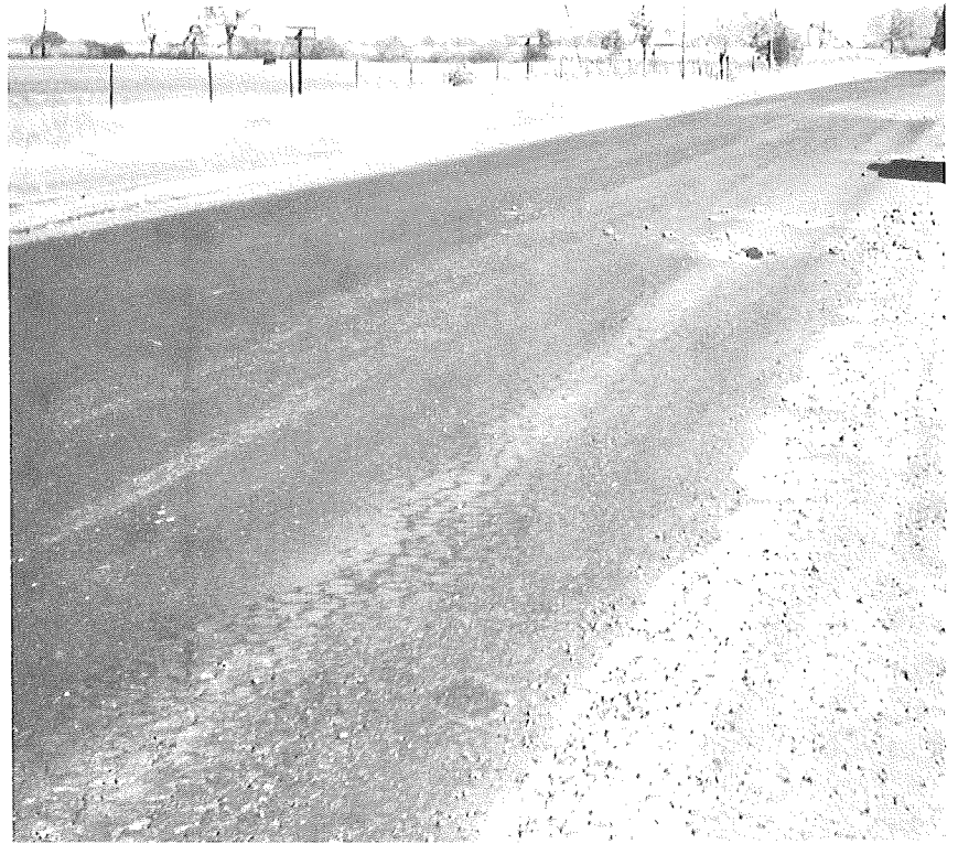
Figure 7. Behavior of asphalt leveling course, showing map cracking and disintegration (upper right), longitudinal cracking and disintegration (lower left) and moisture spotting (lower right).
