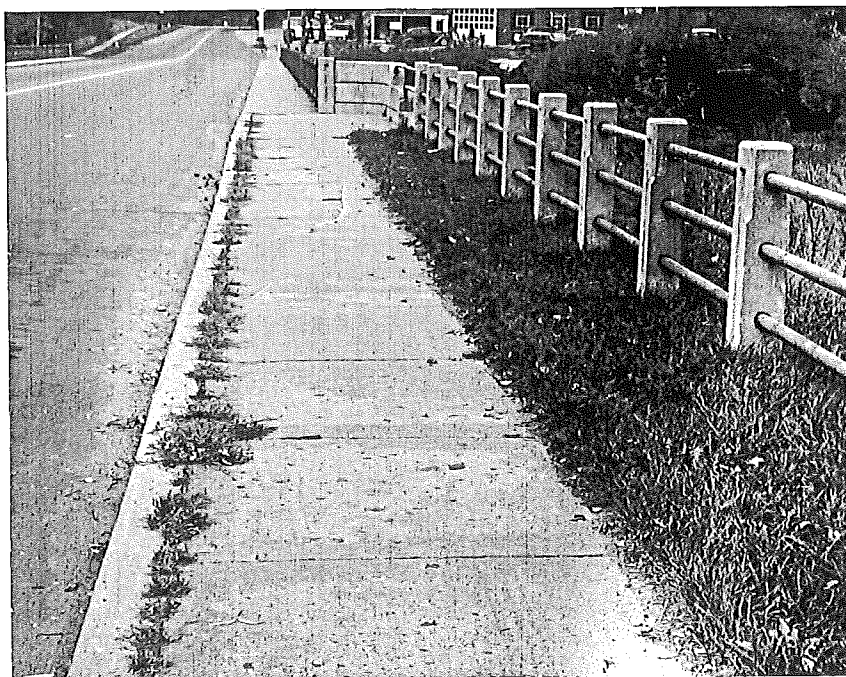
Fig. 6. General view showing scaling of sidewalk, South approach, East side. Standard concrete
