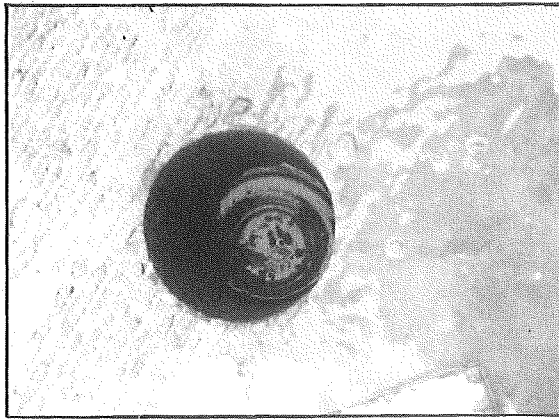
Core hole through pavement showing water retained in the slag base.
