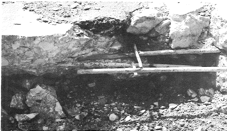
A. Insufficiently lapped wire mesh in the passing lane.
