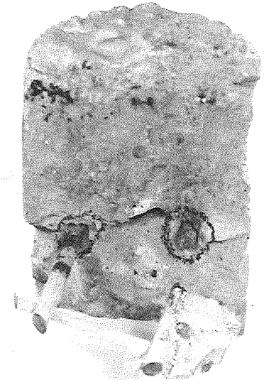
E. Core through passing lane failure crack, broken to show fracture of longitudinal steel.
