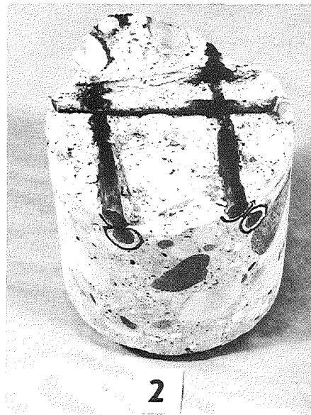
C. Core through section at crosswire in traffic lane, broken at steel level to show failure of crosswire weld.
