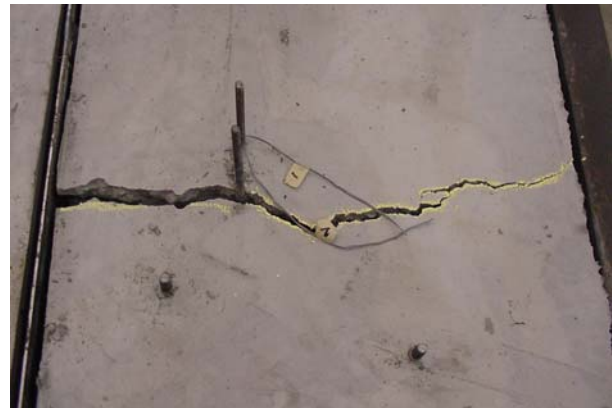
(c) Crack at end of test
