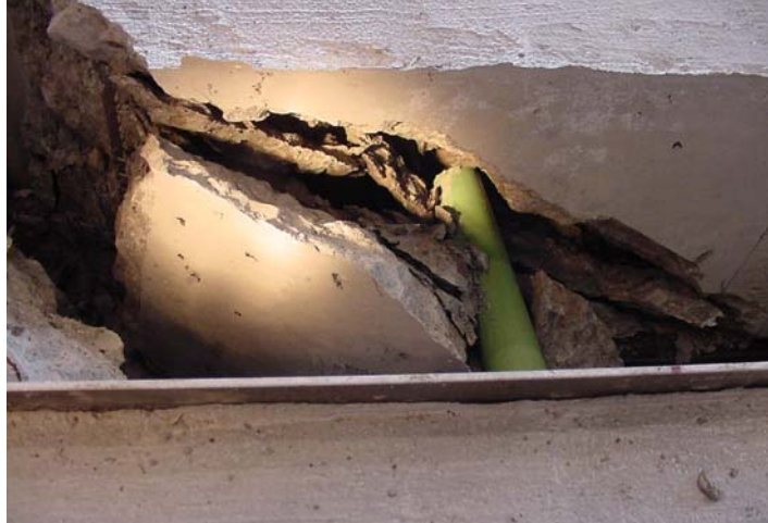
(c) Concrete spalling and cracking around misaligned dowel bar in test specimen
