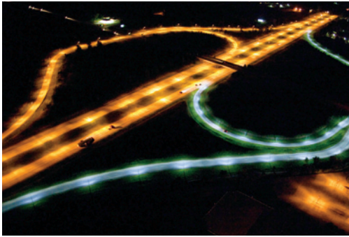
I-275/Eureka Road interchange, west of the Detroit/ Wayne County Metropolitan Airport. Shown at upper left are traditional high-pressure sodium lights (along mainline I-275 in both directions and the northbound ramps), with pilot LED lights shown in the lower right (along the southbound ramps).
