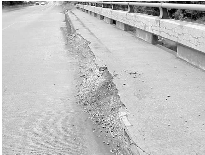
Figure 1: North fascia sidewalk of Mosel Avenue bridge showing deterioration of sidewalk.
