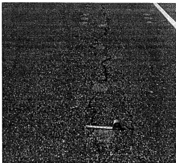
Figure 7.2 A Typical Segregation-Related Cracking at Site 13
