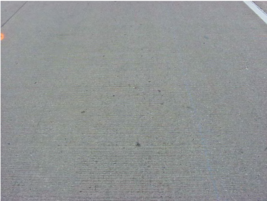
Site 4A: US-23 SB; Starts @ Sta 176+36. Surface of traveling lane showing popouts.
