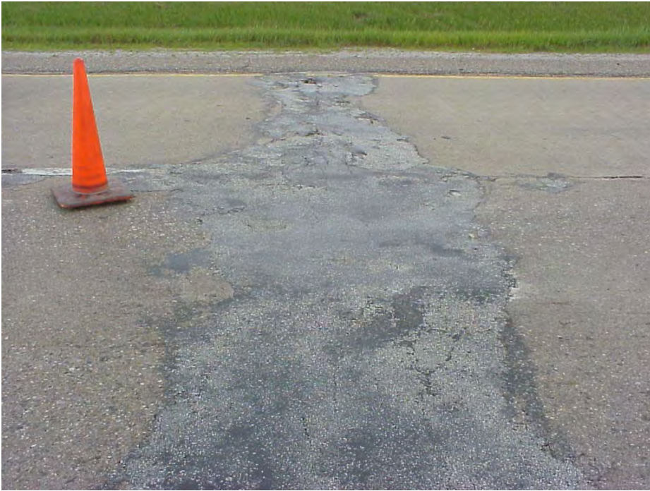
Site 28: US-27 SB Starts @ Station 519+07, View showing the asphalt patching done on transverse joint.
