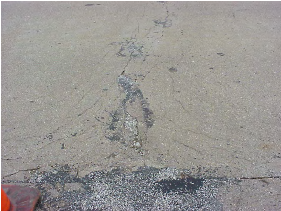
Site 28: US-27 SB Starts @ Station 519+07, View showing the cracking pattern along the transverse cracking.
