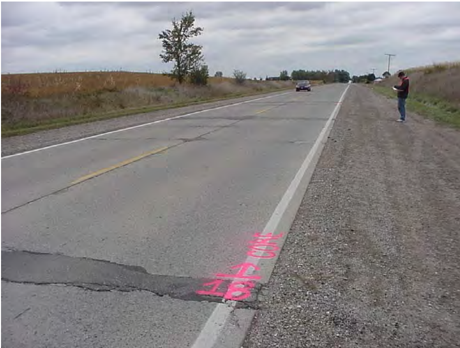
Site 14: M-81 EB. View showing the pavement surface, gravel shoulder and several joint repair patches.
