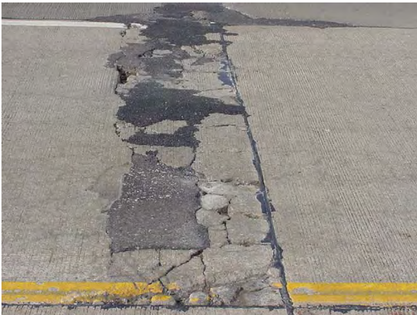
Figure 4. Transverse joint deterioration and map cracking.
