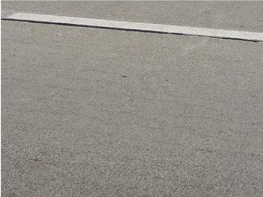
Site 4: US-23 SB, Sta 610+56. Surface of traveling lane showing map cracking.
