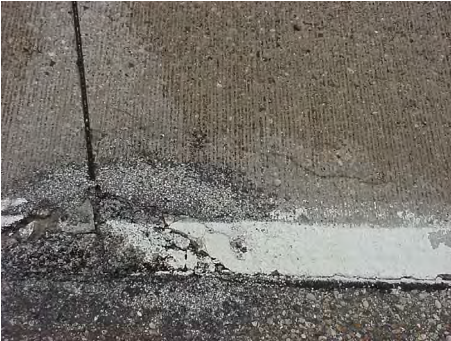
Site 26A: US-10 WB, Sta 137+08. View showing the popouts, cracking pattern and spalling on the pavement. The spalling has already been patched with asphalt.
