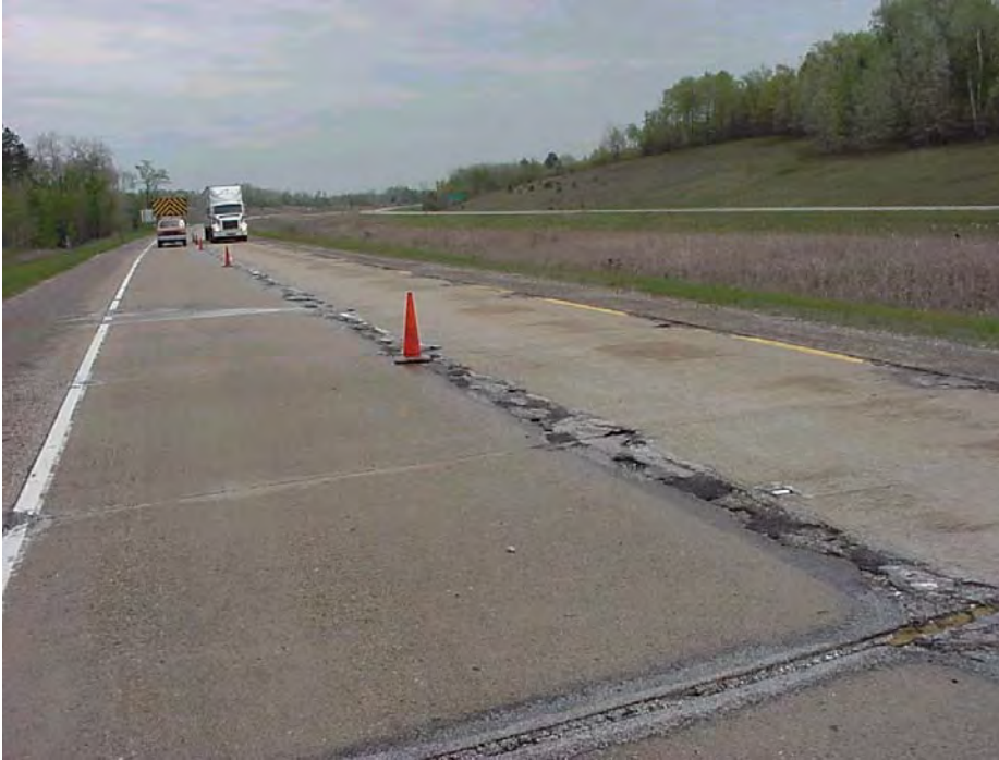
Site 26A: US-10 WB, Sta 137+08. View showing the spalling along the longitudinal joint which has been patched by asphalt. Lower right corner shows a view of expansion joint.
