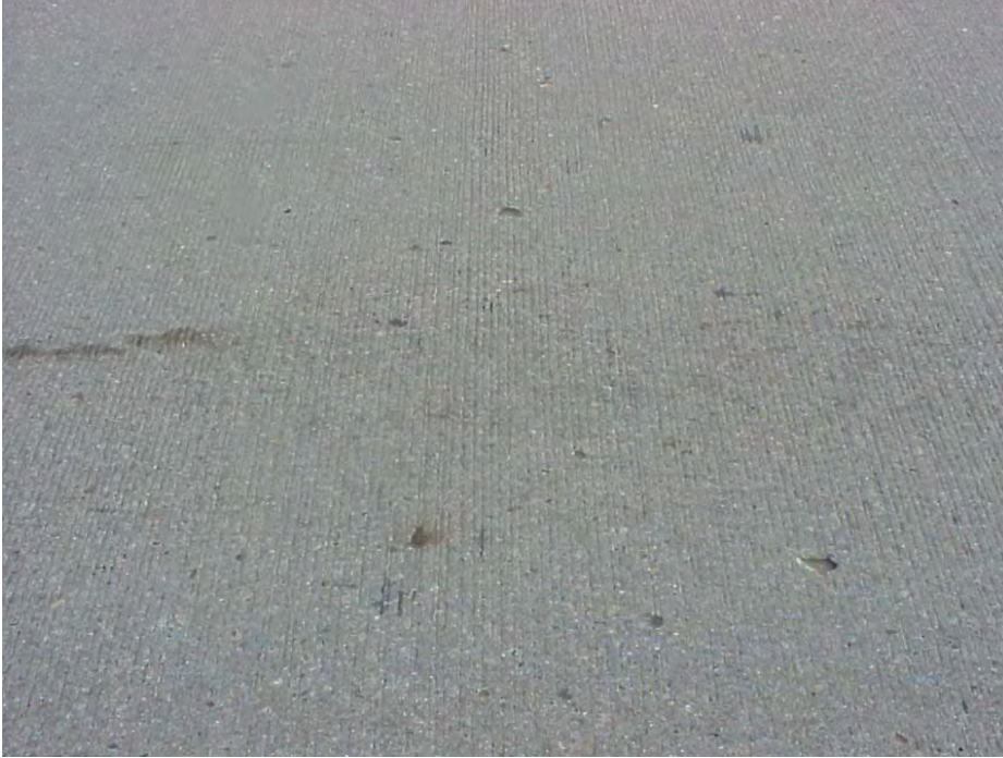
Site 4A: US-23 SB; Starts @ Sta 176+36. Surface of traveling lane-showing Popouts.
