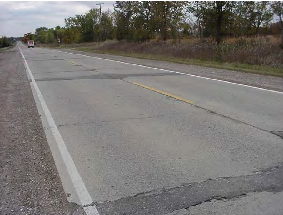
Site 14: M-81 EB. View showing the pavement surface, gravel shoulder, transverse cracks and several joint repair patches.
