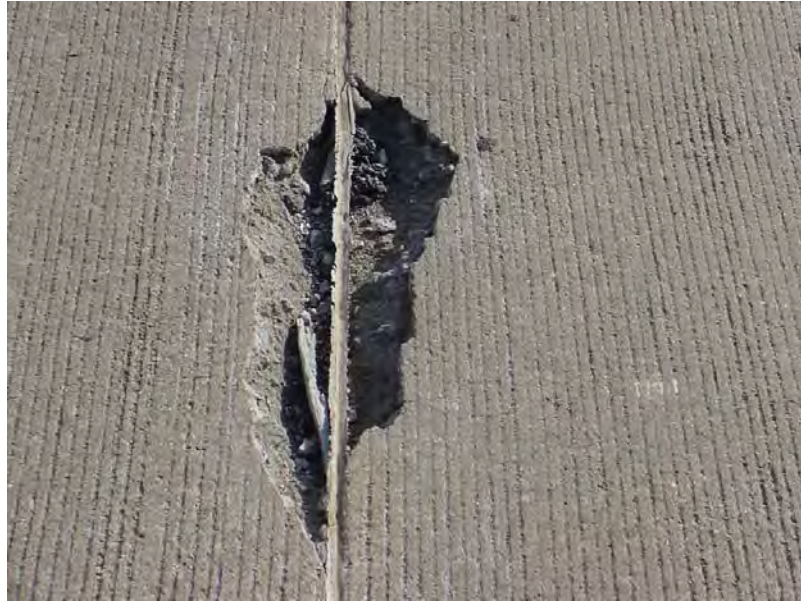
Figure 1. Spall at transverse joint (note paste disintegration).
