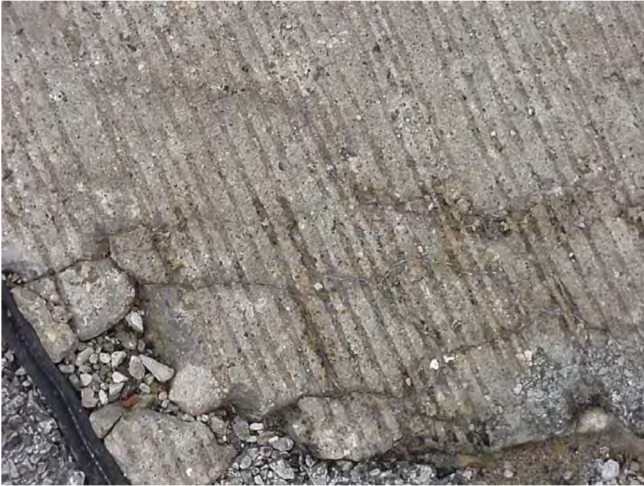
Site 26A: US-10 WB, Sta 137+08. View showing the cracking pattern pavement surface and loose particles.
