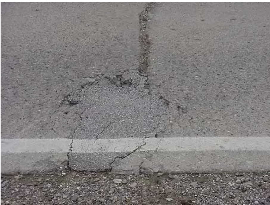
Site 14: M-81 EB. View showing spalling at the end of a transverse crack.
