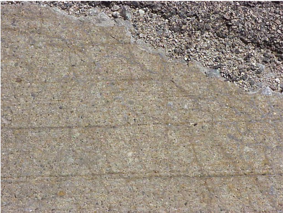
Site 29: I-275 SB, View showing the cracking pattern with white exudate coming out of the cracks (right side of the picture).
