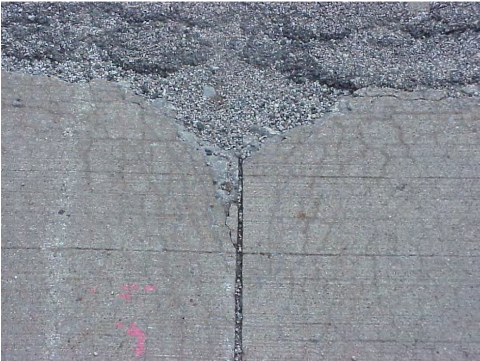
Site 29: I-275 SB, View showing the cracking pattern and asphalt patching at the transverse joint.
