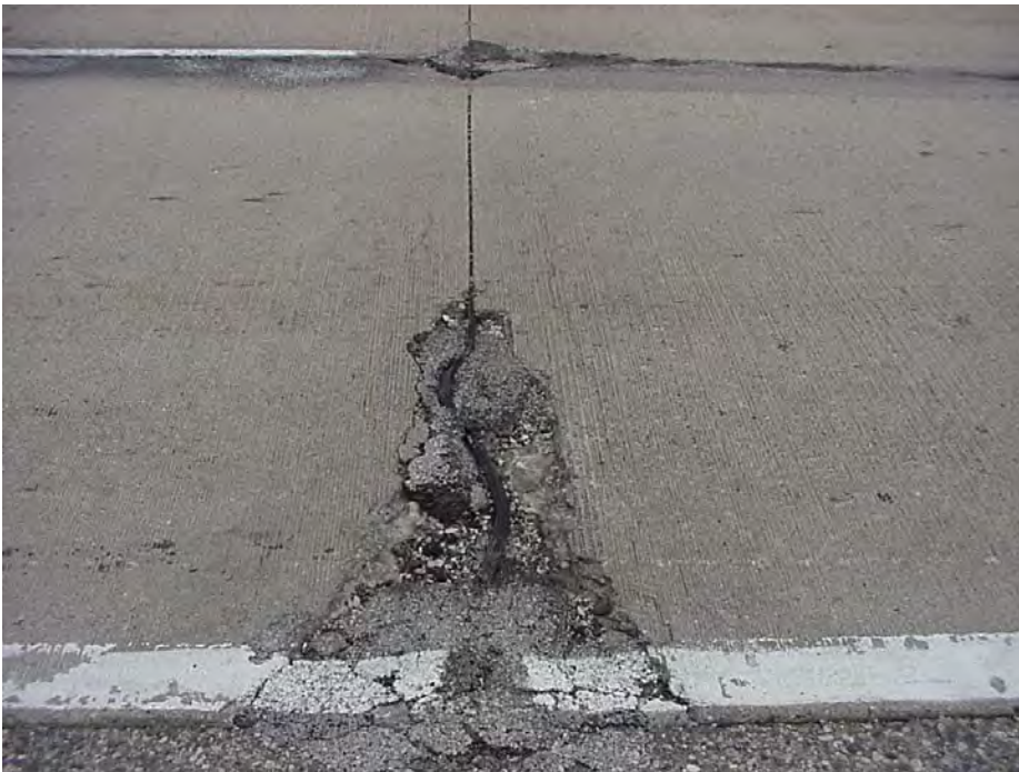
Site 27: US-10 WB, Sta 114+00. View showing the Popouts, cracking pattern and spalled transverse joint.
