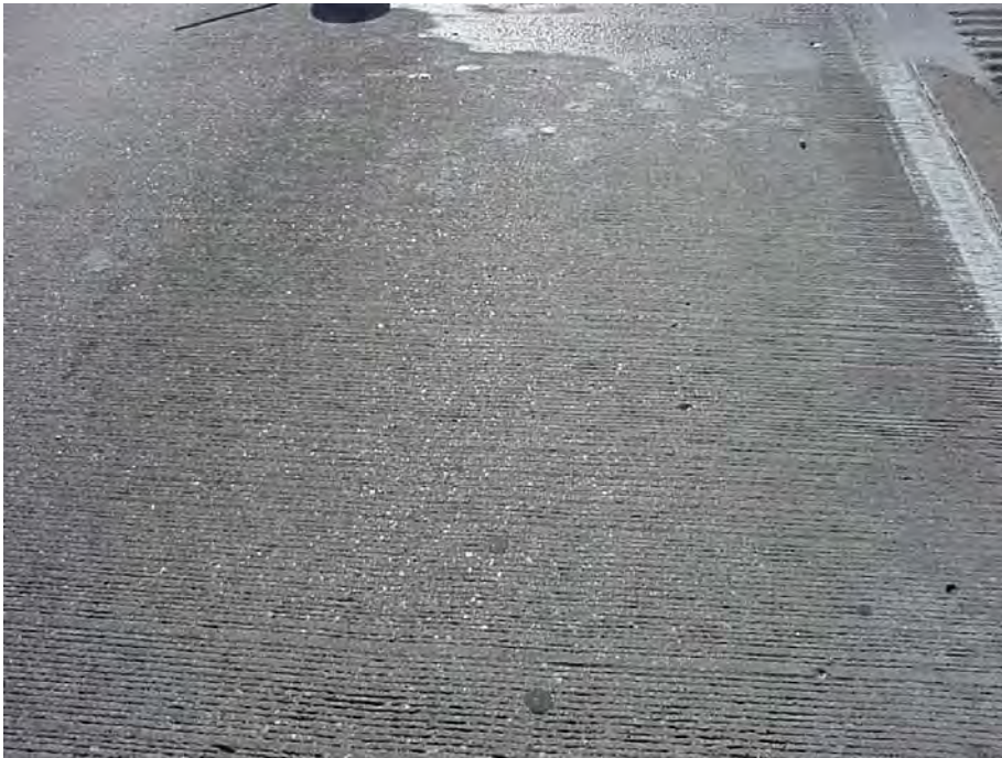
Site 2: US-23 SB, Section C of MDOT Aggregate Study. Surface of traveling lane. Note the popouts in the lower right corner.
