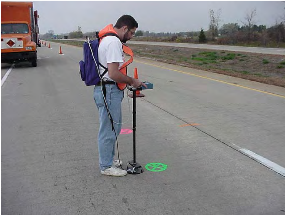
Site 0: US-23 SB, Section A of MDOT Aggregate Study. Permeability testing using the air permeability field apparatus.
