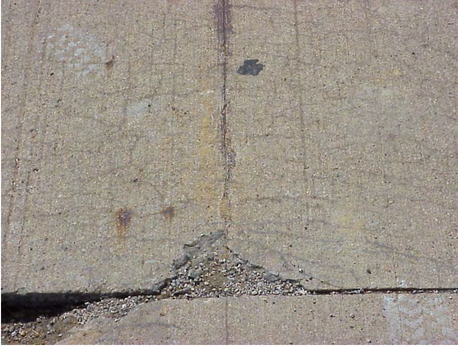
Site 19: M-53 NB @Station 520. Between 17 th and 18 th Mile road, view showing the cracking pattern near a transverse joint.
