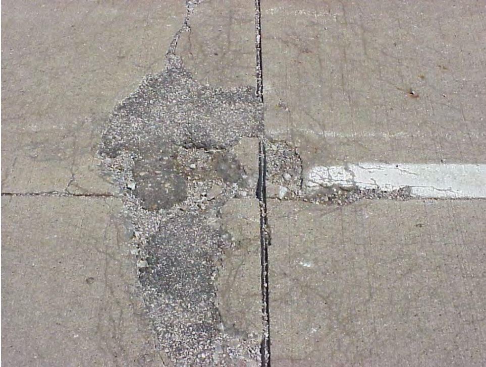
Site 29: I-275 SB, View showing asphalt patching along the transverse joint and also the cracking pattern.
