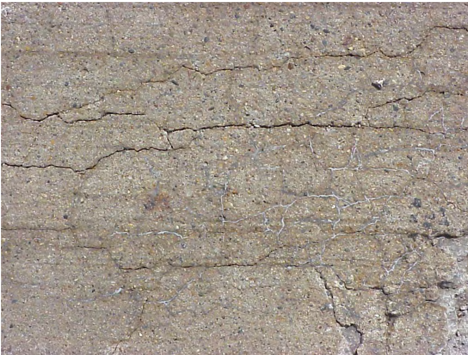
Site 29: I-275 SB, View showing cracking pattern with white exudate coming out of the cracks.
