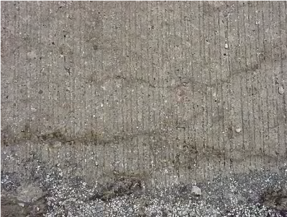
Site 26B: US-10 WB, Sta 137+08. View showing the popouts, cracking pattern and loose particles.
