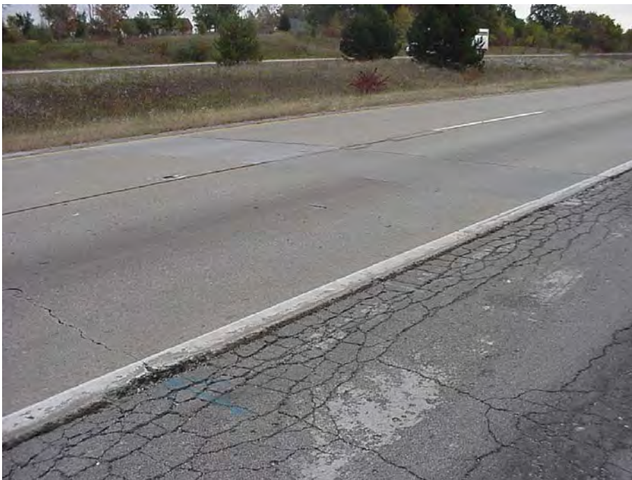
Site 6: I-69 EB, Sta 1534+93. View showing the pavement surface. Note the transverse crack (lower left) and the alligator cracking of the bituminous shoulder.
