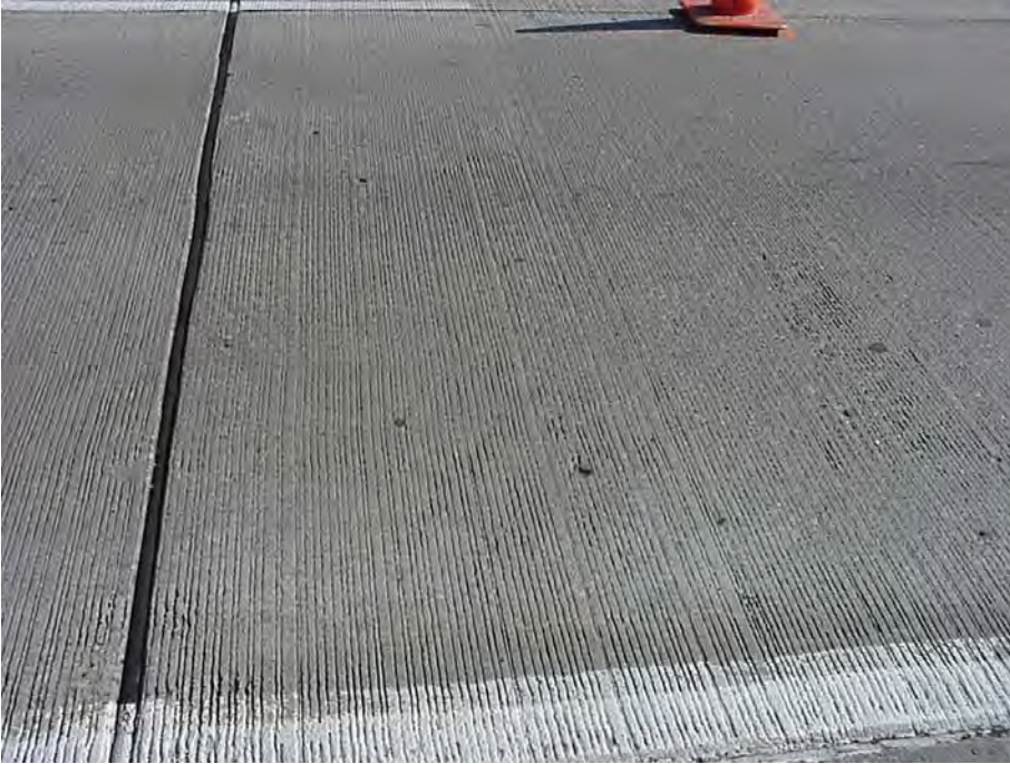
Site 2: US-23 SB, Section C of MDOT Aggregate Study. Surface of outside traveling lane including expansion joint. Note the excellent condition of the joint.
