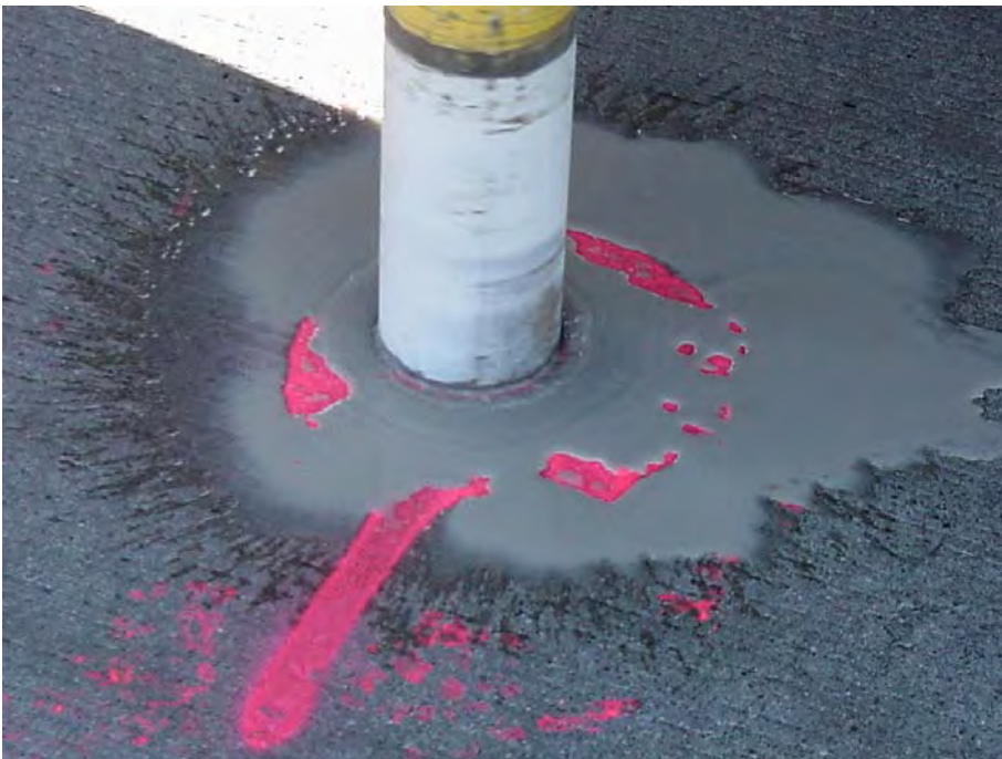
Site 0: US-23 SB, Section A of MDOT Aggregate Study. Coring process for the four-inch core used for permeability and linear traverse testing.
