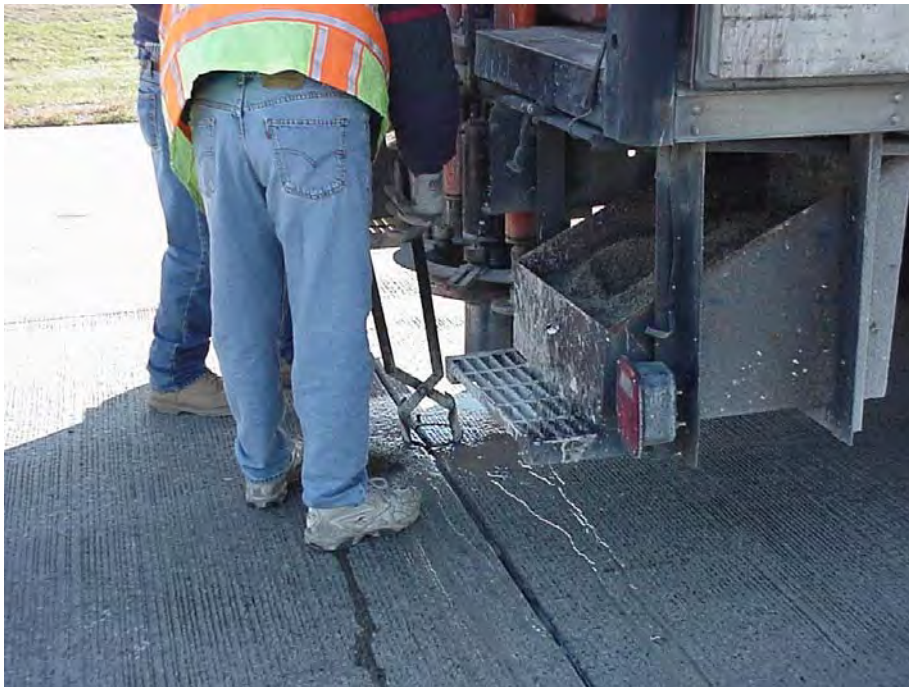
Lower drilling unit used to core the pavement slabs at Site 2, US 23 SB.
