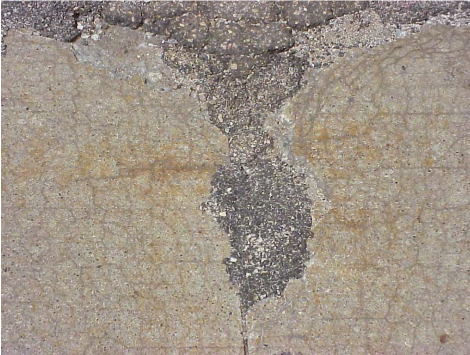
Site 29: I-275 SB, View showing the cracking pattern near the asphalt patching.
