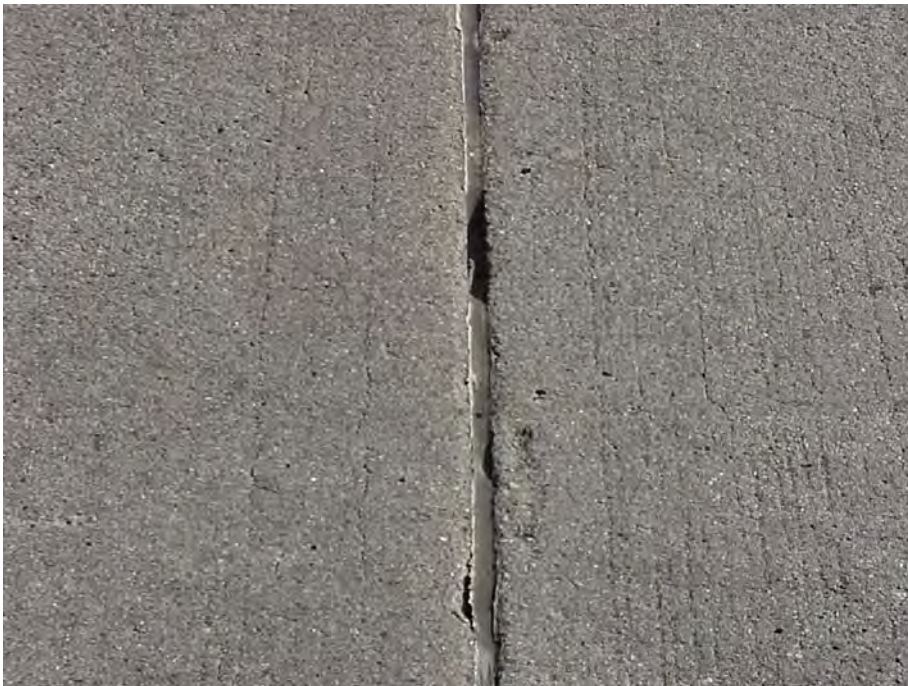
Site 4: US-23 SB, Sta 610+56. Pavement surface and transverse joint. Note the seal of the transverse joint is failing.
