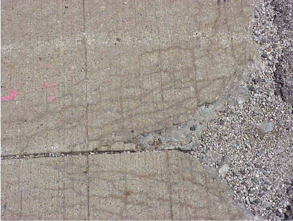
Site 29: I-275 SB, View showing the cracking pattern pavement with white staining coming out of the cracks. Also showing poorly done asphalt patching.
