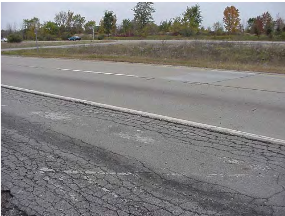
Site 6: I-69 EB, Sta 1534+93. View showing the pavement surface. Note the vertical separation between the traveling lane and the bituminous shoulder.
