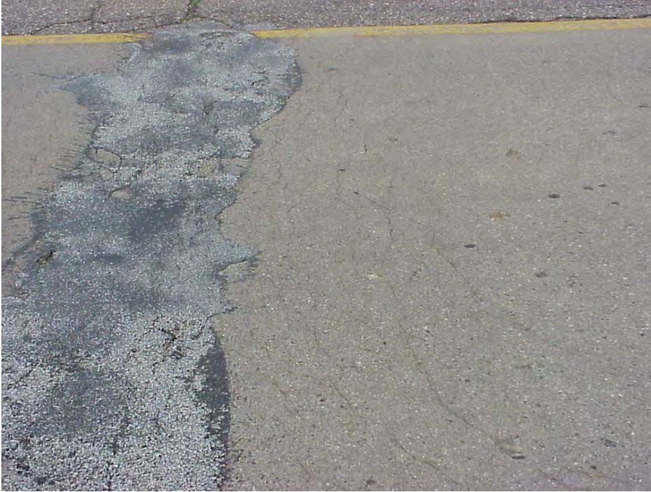
Site 28: US-27 SB Starts @ Station 519+07, View showing the cracking pattern along the poorly done asphalt patching.
