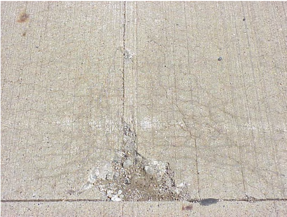
Site 19: M-53 NB @Station 520. Between 17 th and 18 th Mile road, view showing the cracking pattern near a transverse joint.
