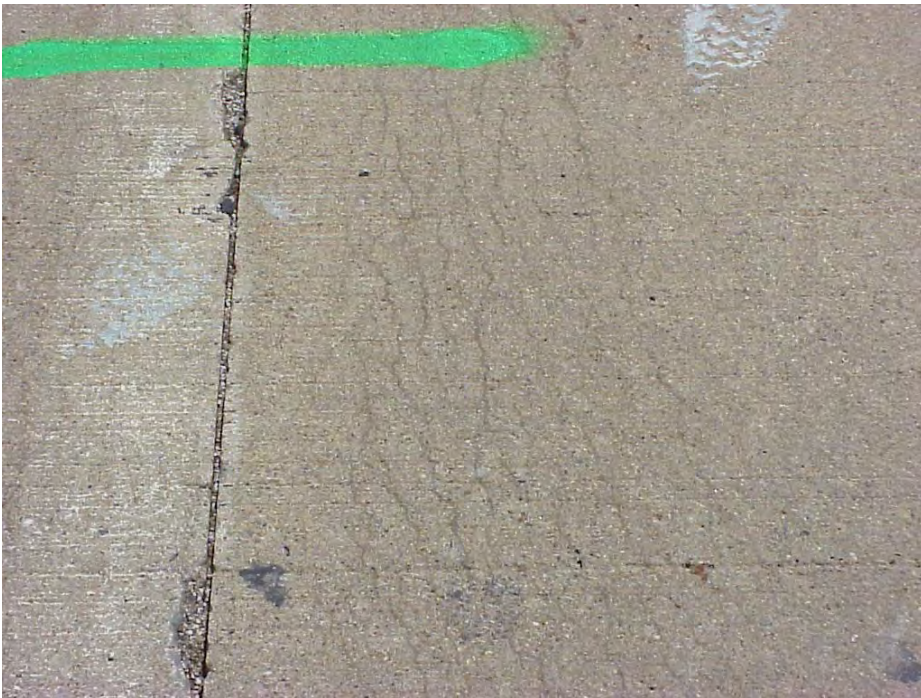
Site 19: M-53 NB @Station 520. Between 17 th and 18 th Mile road, view showing the cracking pattern near a transverse joint
