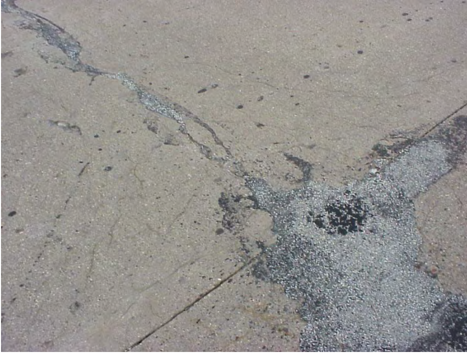
Site 28: US-27 SB Starts @ Station 519+07, View showing the cracking pattern near the longitudinal joint.
