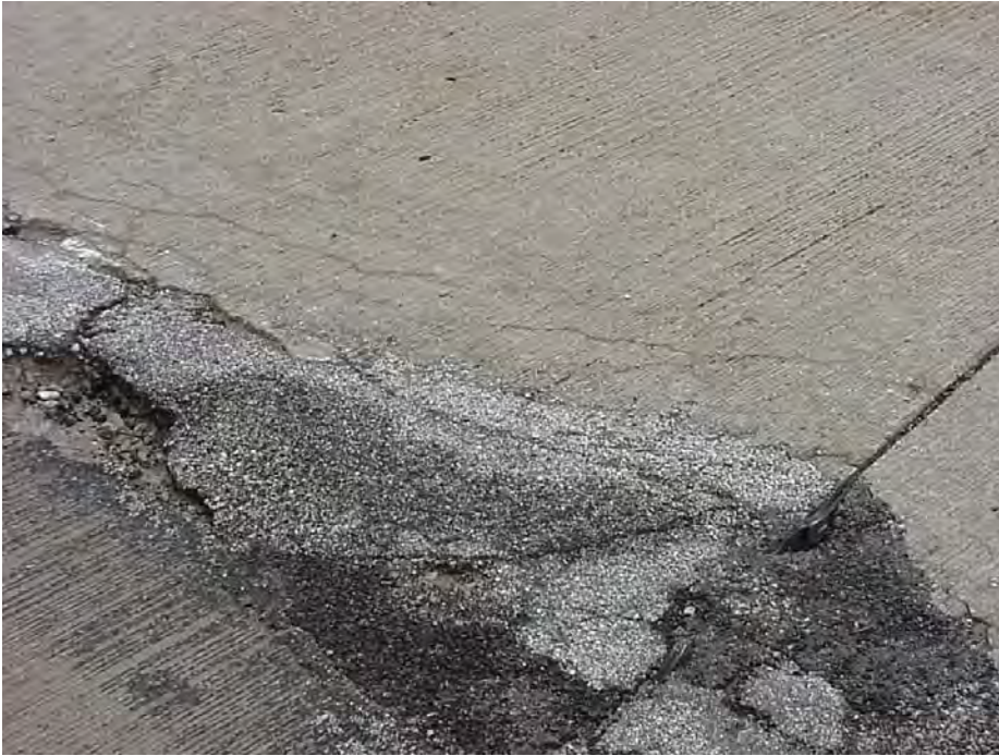
Site 26B: US-10 WB, Sta 137+08. View showing the cracking pattern pavement surface and completely spalled longitudinal joint.
