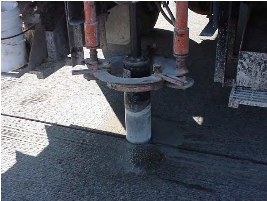
A six-inch joint core is extracted after being drilled. Photo taken at Site 2, US-23 SB.
