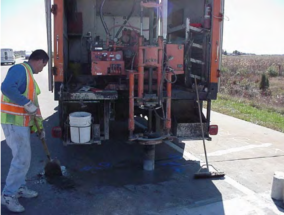
The void from the previous core is filled with a plug (lower right) and mortar while the current core is being taken. Photo taken at Site 1, US-23 SB.
