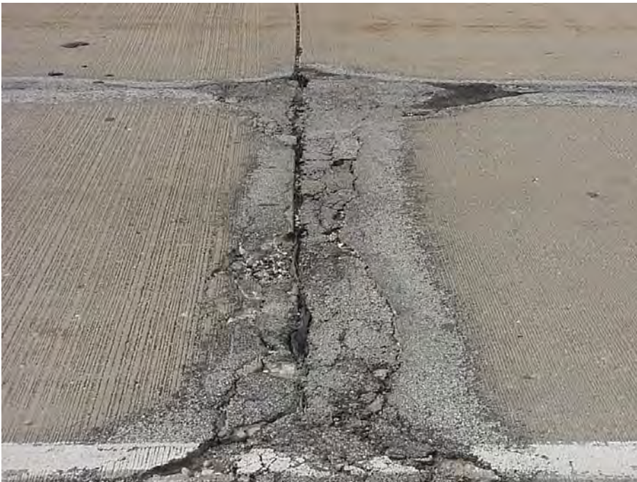
Site 26A: US-10 WB, Sta 137+08. View showing the transverse joint completely spalled and patched with asphalt.
