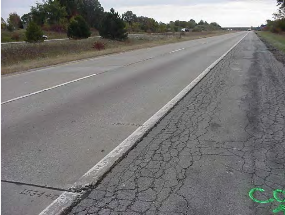
Site 6: I-69 EB, Sta 1534+93. View showing the pavement surface, bituminous shoulder and several concrete patches.
