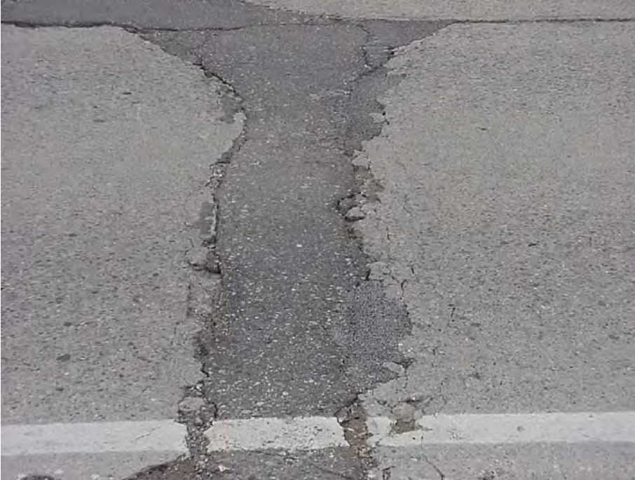
Site 14: M-81 EB. View showing spalling along a severe transverse crack.
