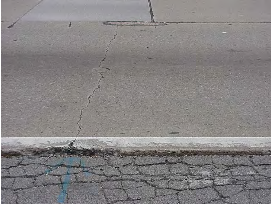
Site 6: I-69 EB, Sta 1534+93. View showing the pavement surface. Note the transverse crack, concrete patch, and the spalling at the lower right edge of the concrete patch.
