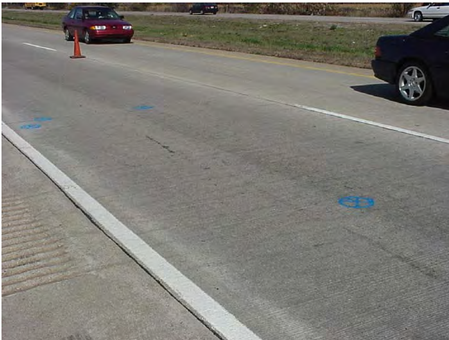
Site 3: US-23 SB, Section D of MDOT Aggregate Study. Surface of traveling lane showing the position of the six-inch cores. Note the shrinkage cracking throughout the site.
