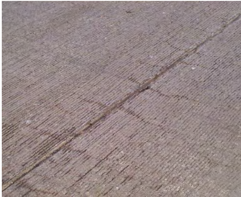
Figure 2. Cracking running perpendicular to transverse joint.
