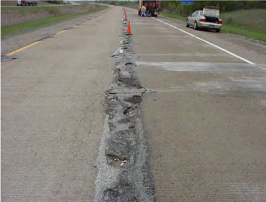
Site 26B: US-10 WB, Sta 137+08. View showing spalling along the longitudinal joint which has been patched by asphalt.
