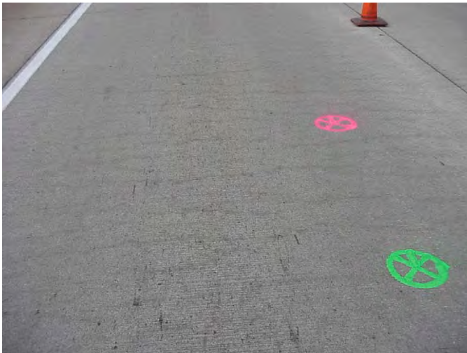
Site 0: US-23 SB, Section A of MDOT Aggregate Study. Four-inch core locations. Note the presence of shrinkage cracking in test slab.
