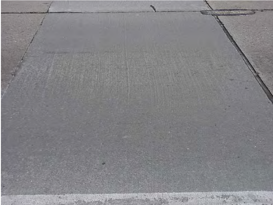
Site 6: I-69 EB, Sta 1534+93. View showing a concrete patch. Note the expansion joint on the right side of the patch and the spalling at the upper right corner.
