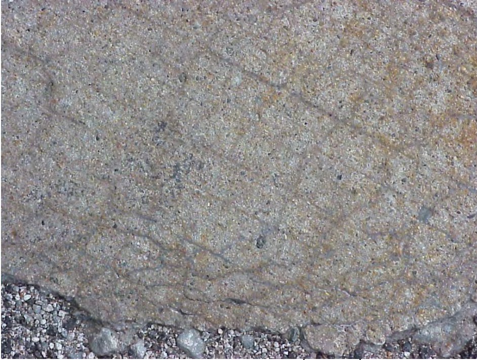
Site 19: M-53 NB @Station 520. Between 17 th and 18 th Mile road, view showing the cracking pattern near a transverse joint.
