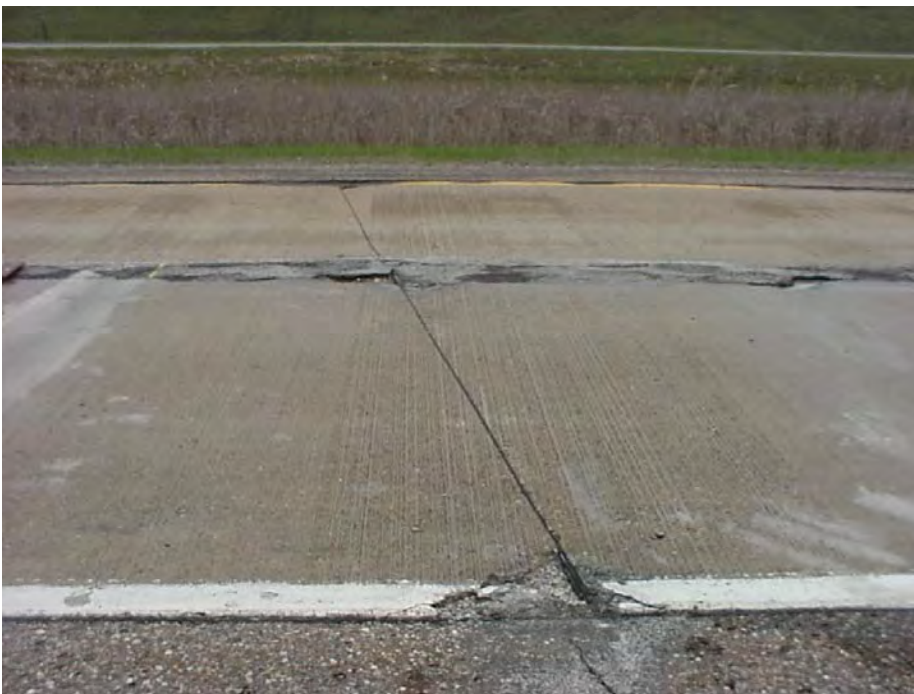
Site 26B: US-10 WB, Sta 137+08. View showing the skewed joint. Also showing spalling at the corners of joint.
