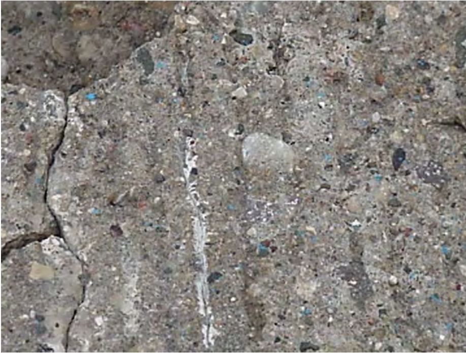
Site 27: US-10 WB, Sta 114+00. View showing the cracking pattern on pavement surface with breakup of the pavement.
