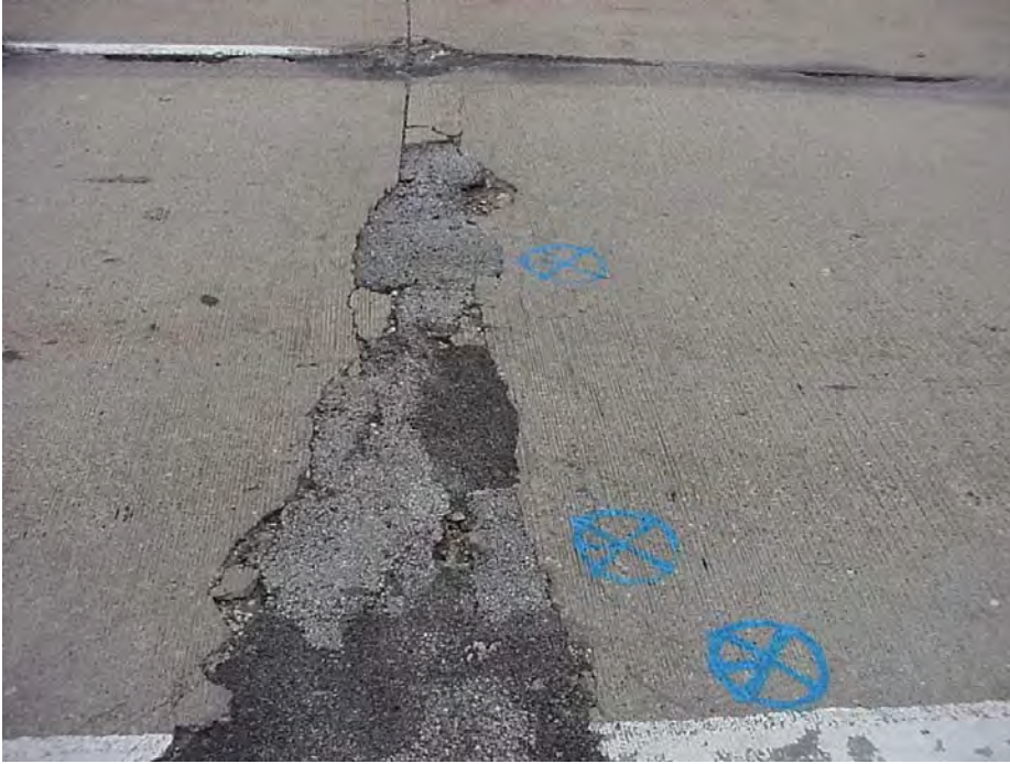
Site 27: US-10 WB, Sta 114+00. View showing spalling along the transverse joint and coring locations for petrographic analysis.
