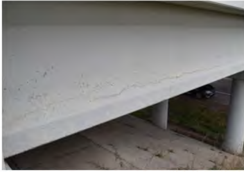
(a) Bottom flange longitudinal cracking
