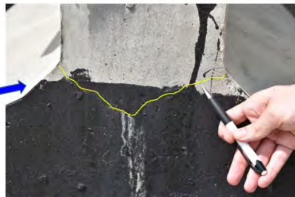
Close-up views of the crack with efflorescence at the bottom of the web
