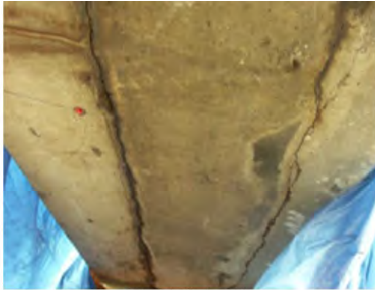
(a) Longitudinal cracking
