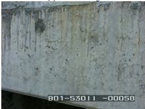
(c) Map cracking on exterior girder web
