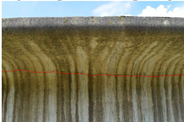
Longitudinal crack at the top of the web
