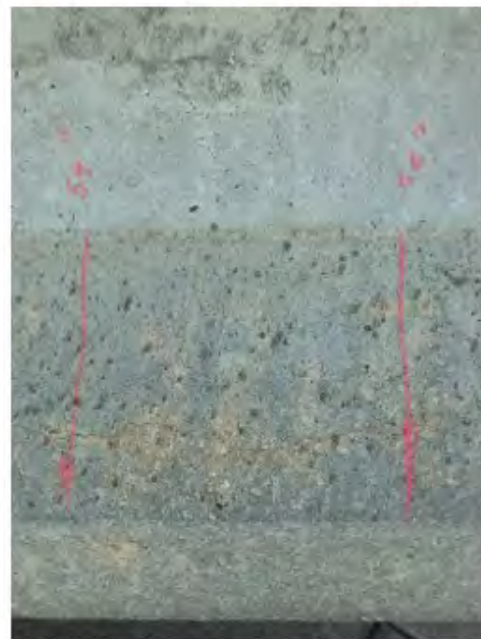
(c) Outside surface of the bottom flange
