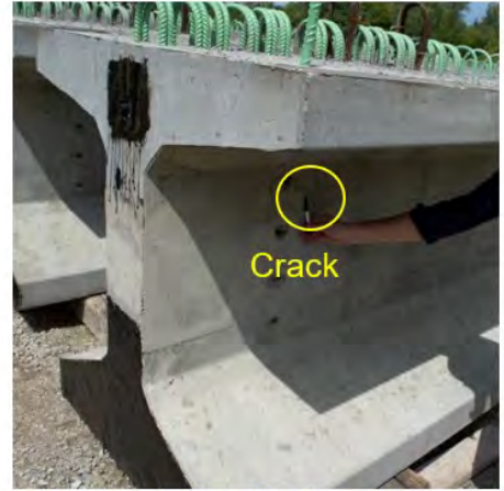
Isometric view showing a diagonal crack on the web
