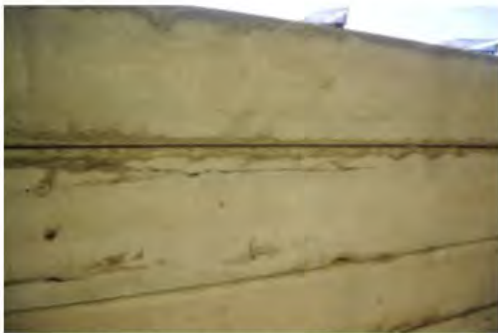
(a) Longitudinal cracks in box-beam bottom flange (Frosch et al. 2020a)
