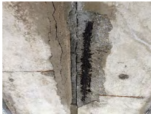
(c) A close-up view of a deteriorated beam
