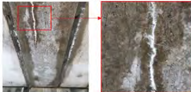
(e) Heavy random cracking (Cracking-PSC 1110) Condition State 4
