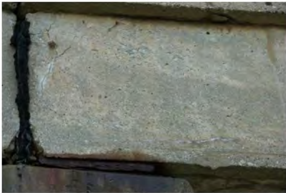
(a) End cracking
