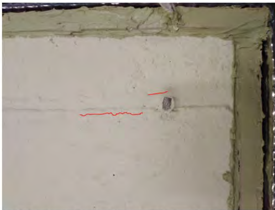
(a) Initial cracks in Si-Rex 03 applied slabs before exposed to 120° F. Red color line represents the cracks in the coating.
