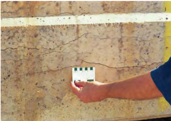
b) PC box beam cracking
