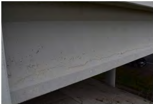
(c) Wide longitudinal cracking (Cracking-PSC 1110), Condition State 3
