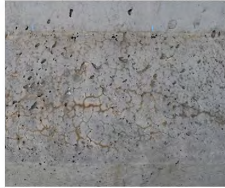
(b) Heavy map cracking on bottom flange (Cracking-PSC 1110), Condition State 2
