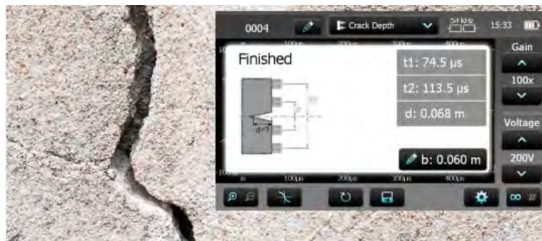
Figure 2-49. Crack depth calculation using Proceq Pundit PL-200 data (Proceq 2014)
