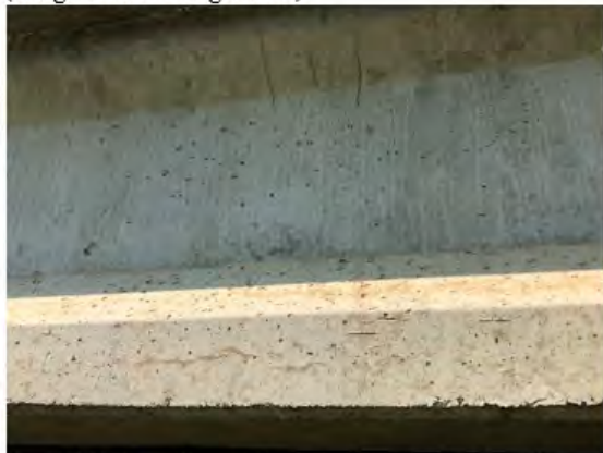
(c) Bottom flange showing longitudinal cracks
