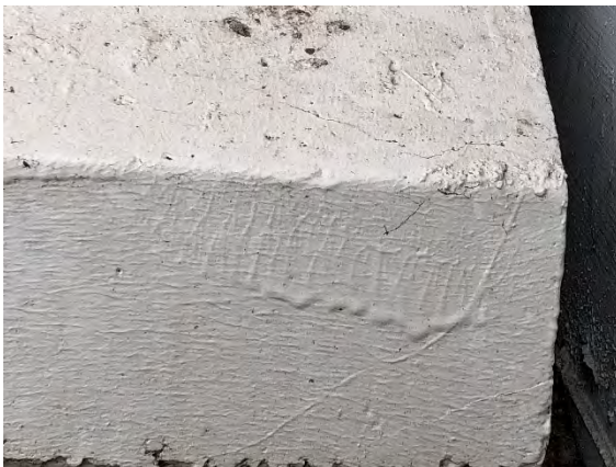
(c) Exposed cracks on top of the bottom flange
