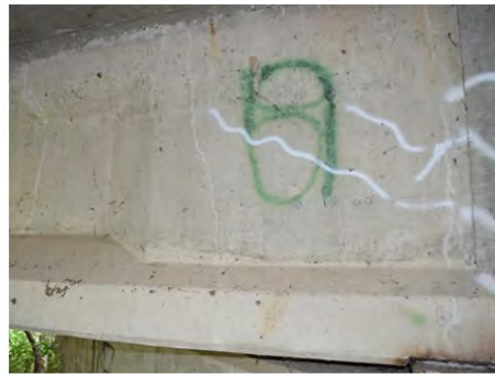
(b) Diagonal cracking – From girder bottom to girder top
