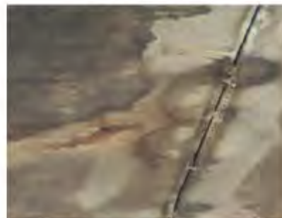
(g) Heavy build-up with rust staining. (Efflorescence / Rust Staining 1120) Condition State 3
