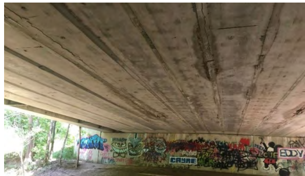
(b) Moist shear keys and longitudinal cracking
