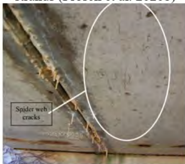
(e) Spider web cracks in box-beam bottom flange (Frosch et al. 2020b)
