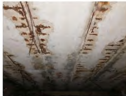
(b) Spalling, corrosion, and broken prestressing strands in box-beams (Frosch et al. 2020a)
