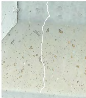
(a) Vertical cracking
