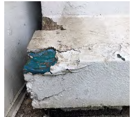
c) Beam end cracking
