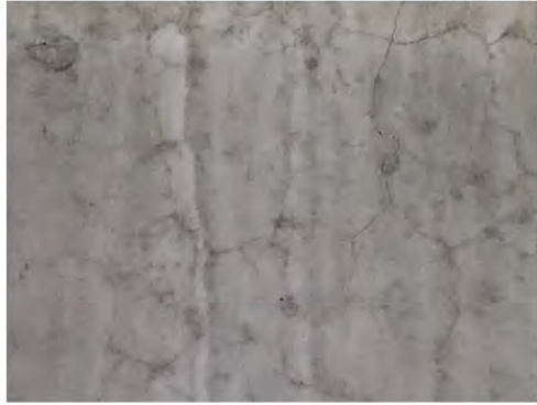
(a) Heavy map cracking on web (Cracking-PSC 1110), Condition State 2
