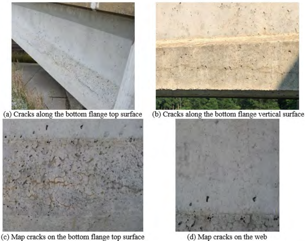
Figure 3-9. Map and longitudinal cracks in PSC I-beams
