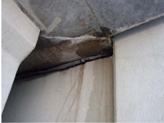
Figure 2-12. Cracking of Minnesota bridge deck at the reentrant corner
