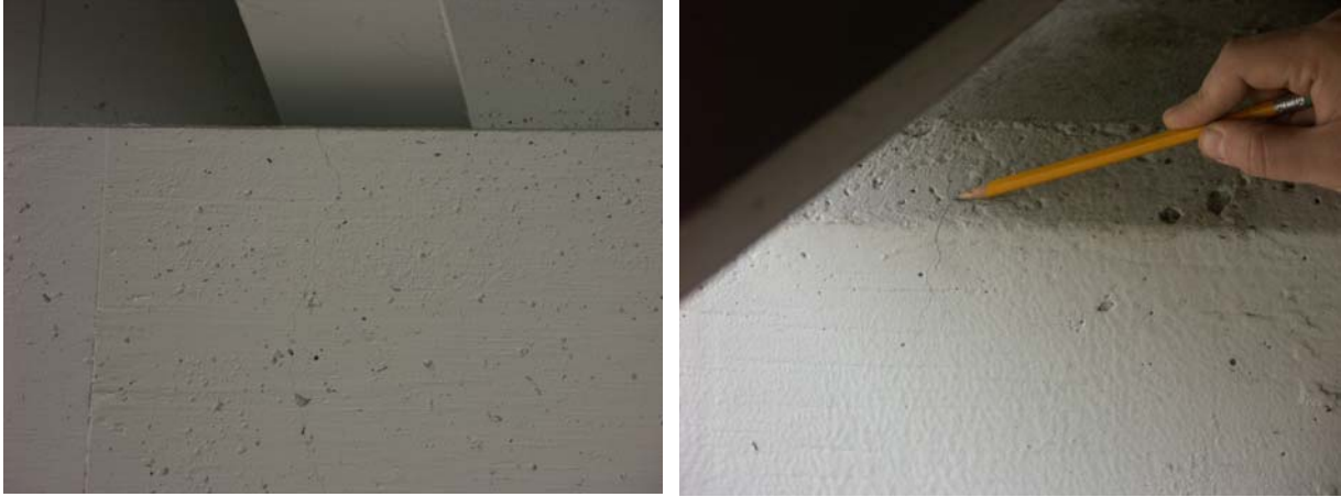
Photo C - 10. Abutment wall cracking
