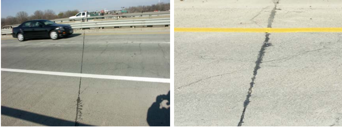
Photo C - 19. Saw cut provided on the link slab over the pier (I-69 EB)
