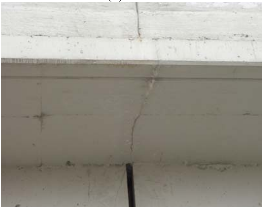
(b) Full depth link slab cracks – deck overhang North Bound
