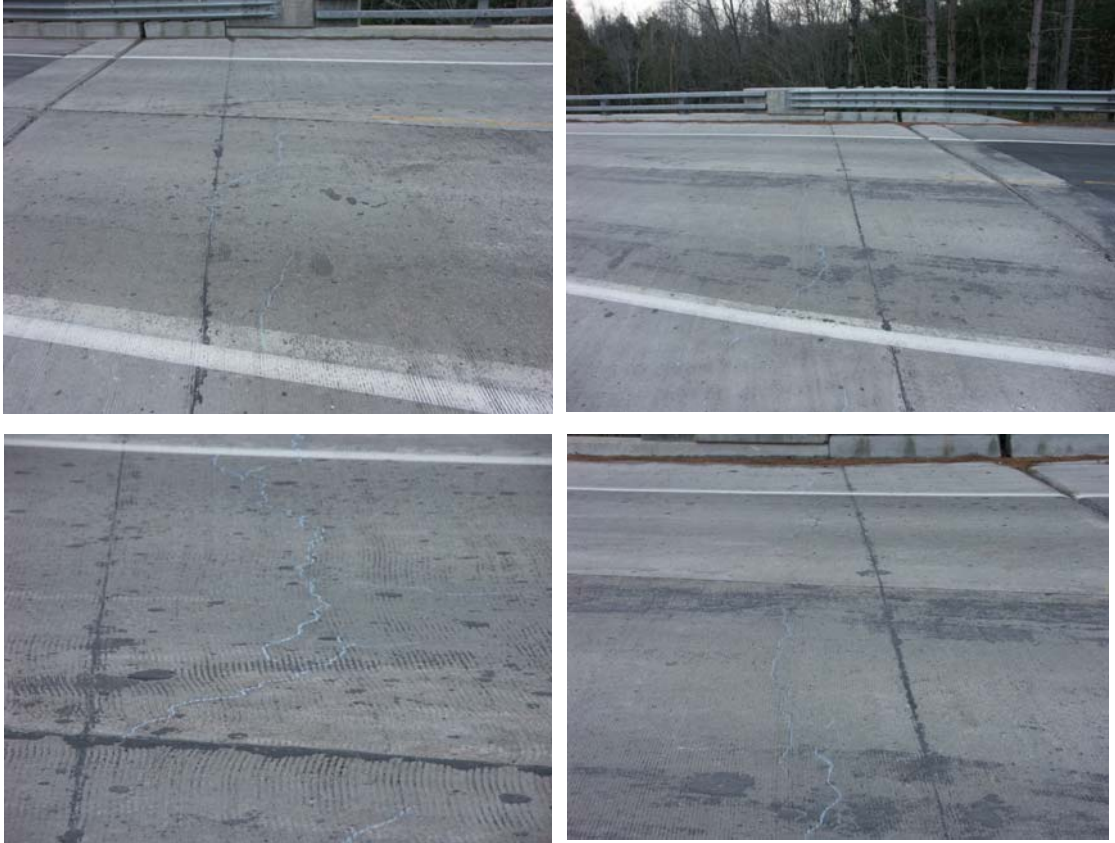
Photo C - 14. Approach slab cracking
