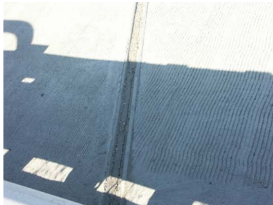
Photo C - 21. Debris filled joint with cracks (I-69 EB)
