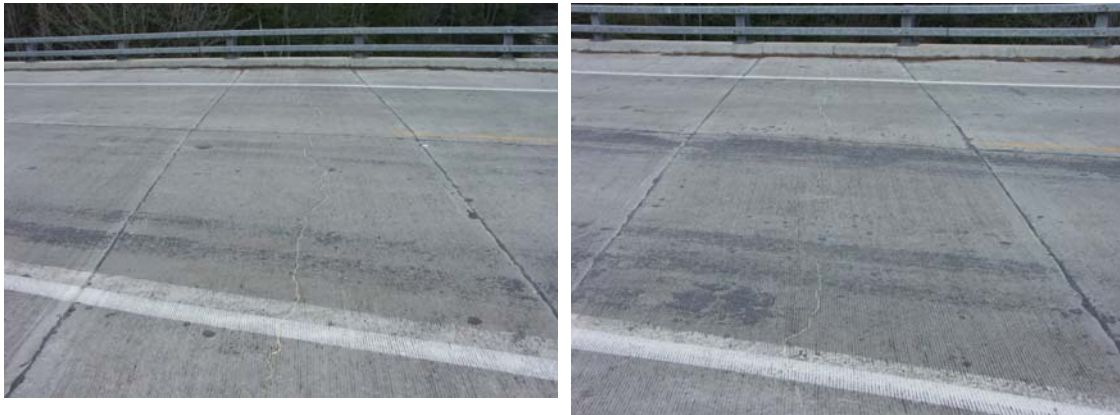
Photo C - 13. Link slab cracking
