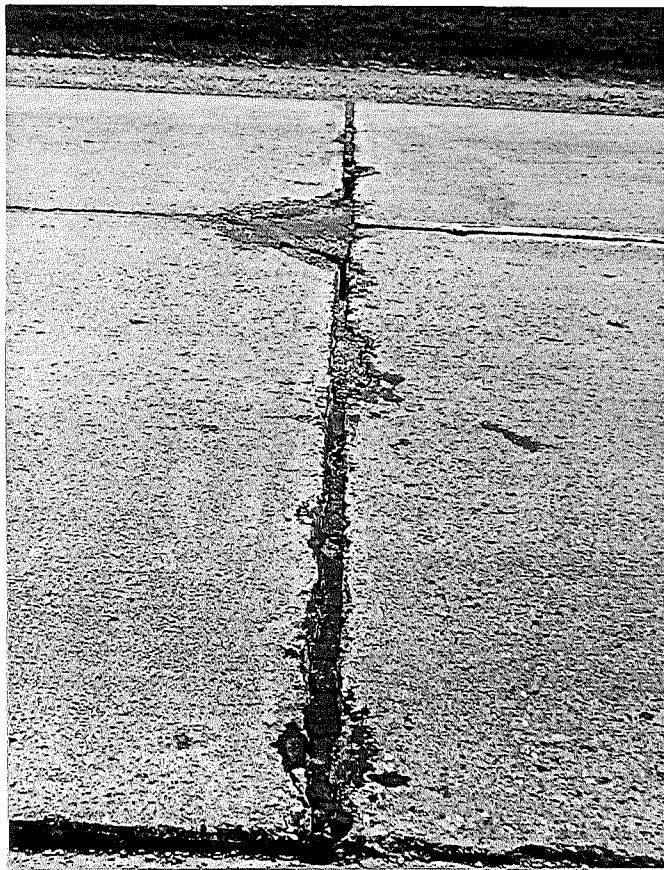
Figure 1. Joint resealed with hot-pour where original preformed sealer had disappeared. Note spall and center-joint break (Sta 249+30).
