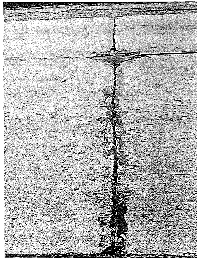
Figure 2. Test joint showing some re-sealing with hot-pour where original preformed sealer was torn and ragged (Sta 248+70).
