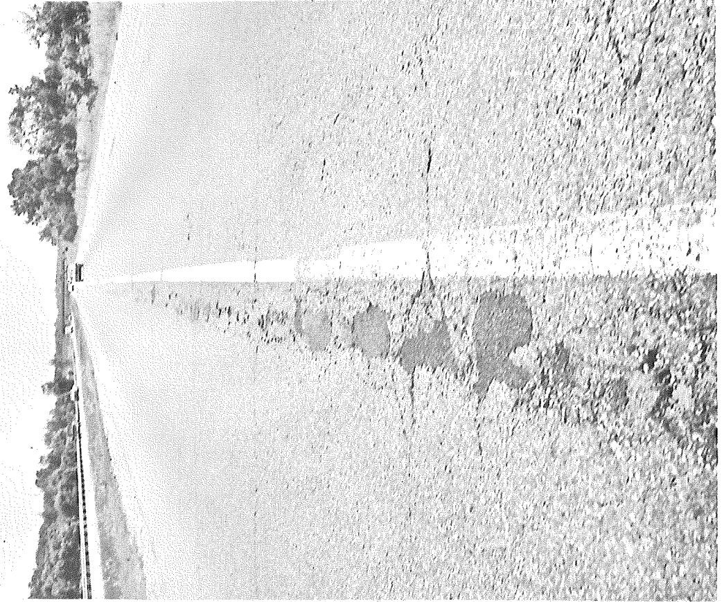
Figure 7 (below). Deterioration along reflection crack, on east-bound roadway.
