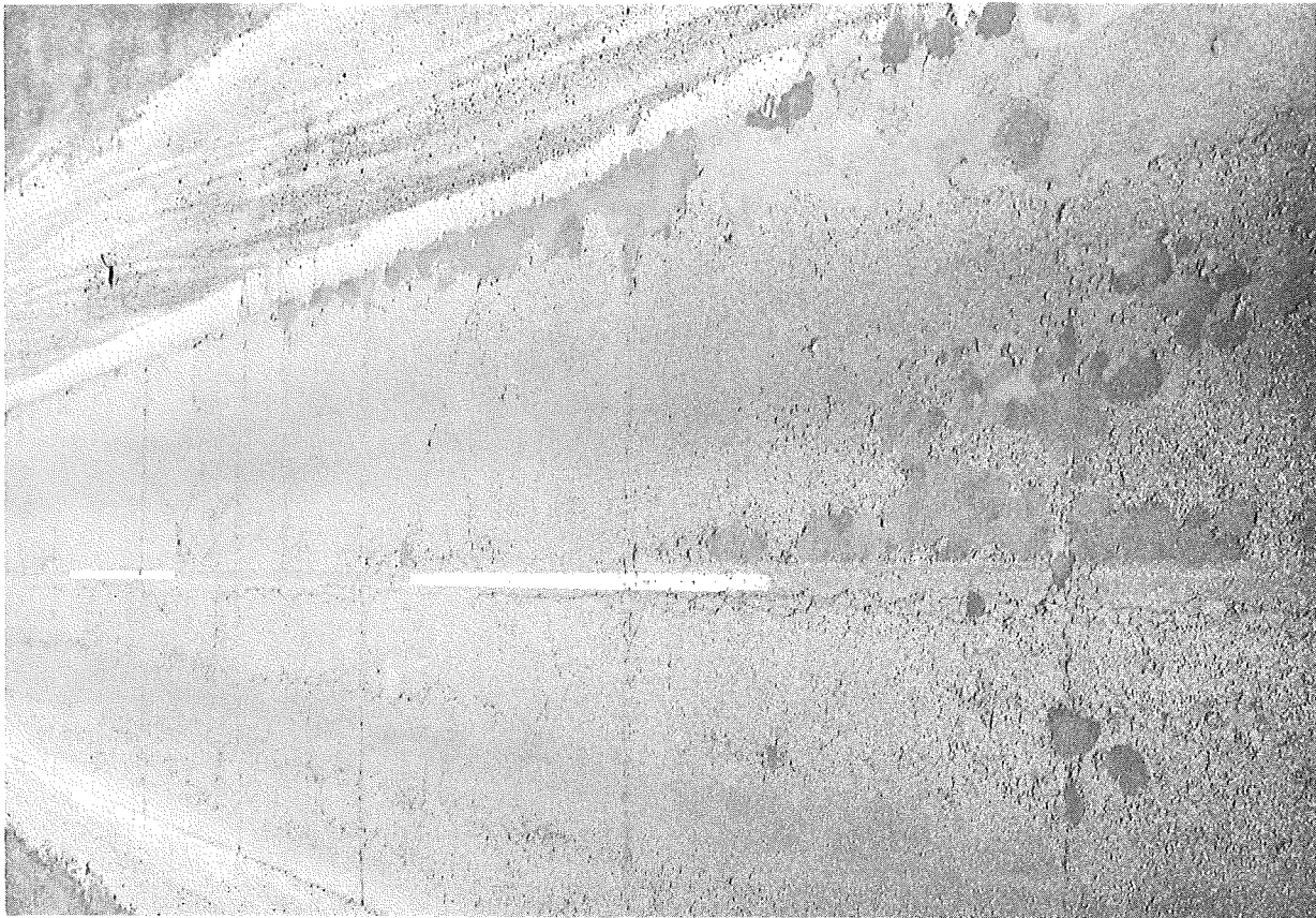
Figure 4. Advanced deterioration in evidence over a large portion of reinforced bituminous surface.
