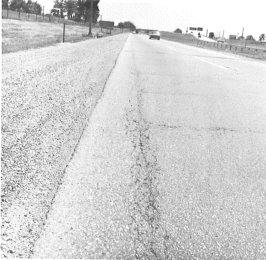
Figure 2 (left). Typical reflection cracking over the longitudinal widening strip joint.
