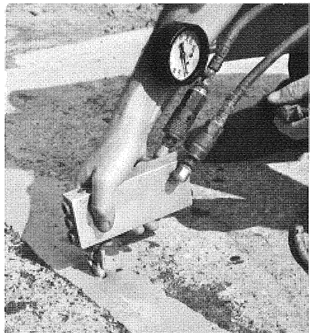
Figure 10. Close-up of mixing nozzle and pressure gage.
