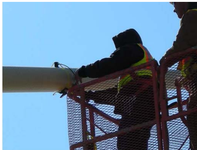
Figure C-9. Mounting of an AE sensor on a bridge cable (Parmar and Sharp 2009)
