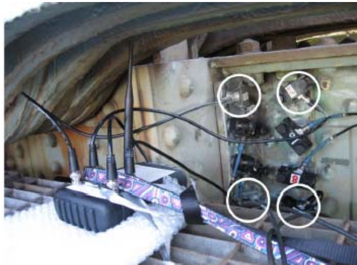
Figure C-12. The monitoring systems wired and wireless (marked in circles) AE sensors (Ledeczi et al. 2009)
