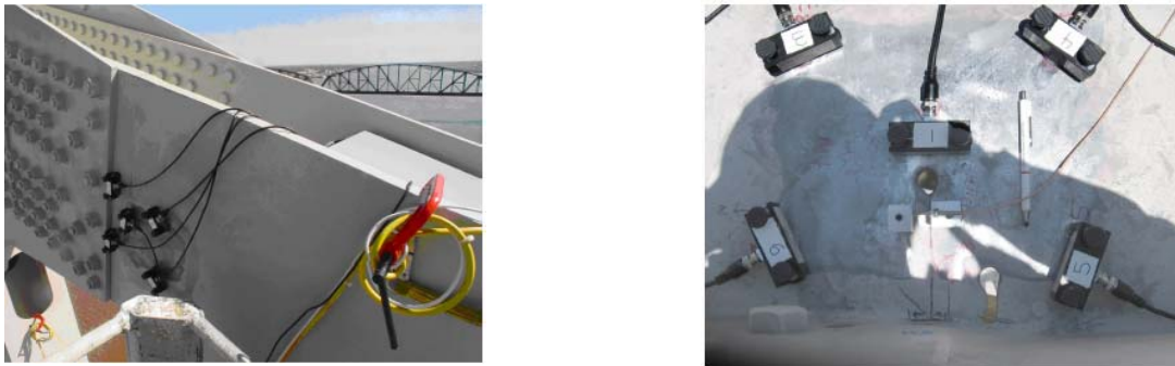
Figure C-8. Field monitoring of a fatigue crack using an AE sensor array (Kosnik 2008)
