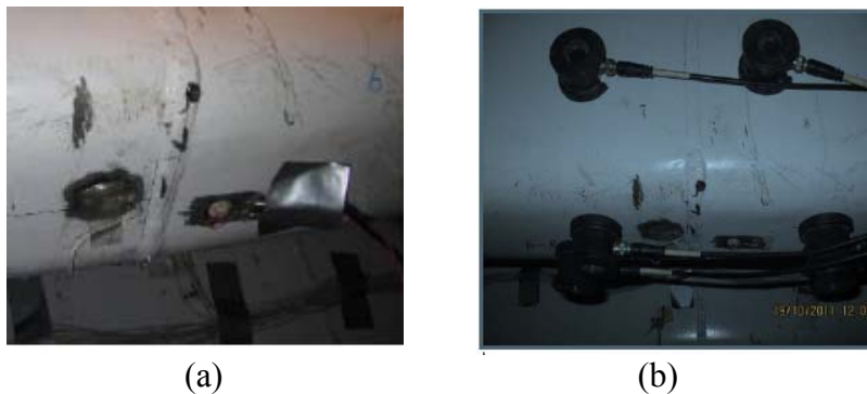
Figure C-14. Sensors mounted near the weld joint of the structure (a) strain gauges and PZT paint sensors and (b) commercial AE sensors (Yi et al. 2012)
