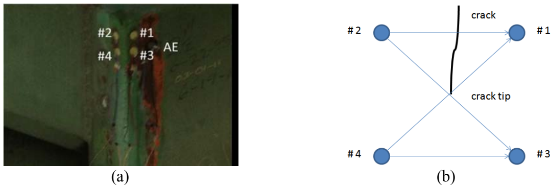
Figure C-3. Field implementation of the system for fatigue crack monitoring (a) sensor system mounted on the bridge and (b) schematic of the USGW sensor array (Zhao et al. 2013)
