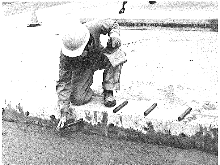
Inserting 1-3/16-in. diameter by 9-in. long steel dowels in holes for precast slab repair.
