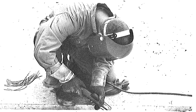
Welding dowels to steel plate. Note welding rods are about in semi-circle to facilitate welding the lower half of dowel to the plate.
