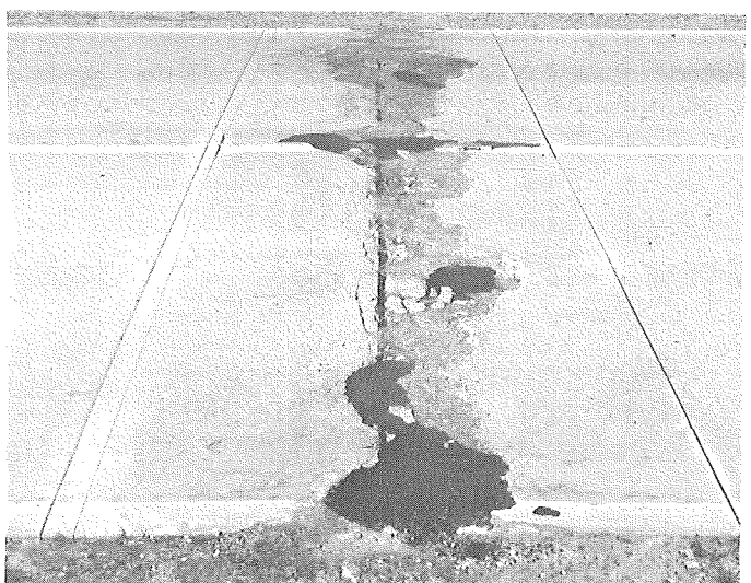
Overall view of sawed repair area. Note narrowly spaced saw cuts in the left of photo.
