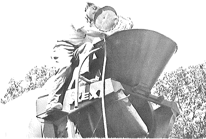
Adding calcium chloride to concrete mix at repair site to accelerate early strength gain.
