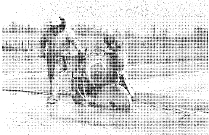
Full-depth sawing of 9-in. concrete pavement using 65-hp saw equipped with 26-in. diameter diamond blade.
