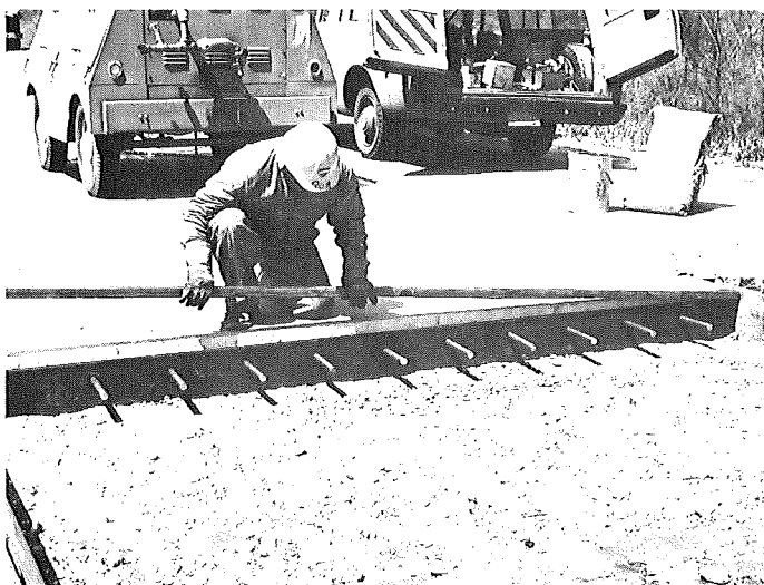
Doweled expansion joint being readied at cast-in-place repair site. The filler is bituminous impregnated filler board.
