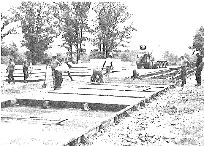
Pouring and finishing slabs. Twenty to twenty-five slabs were cast at one time.
