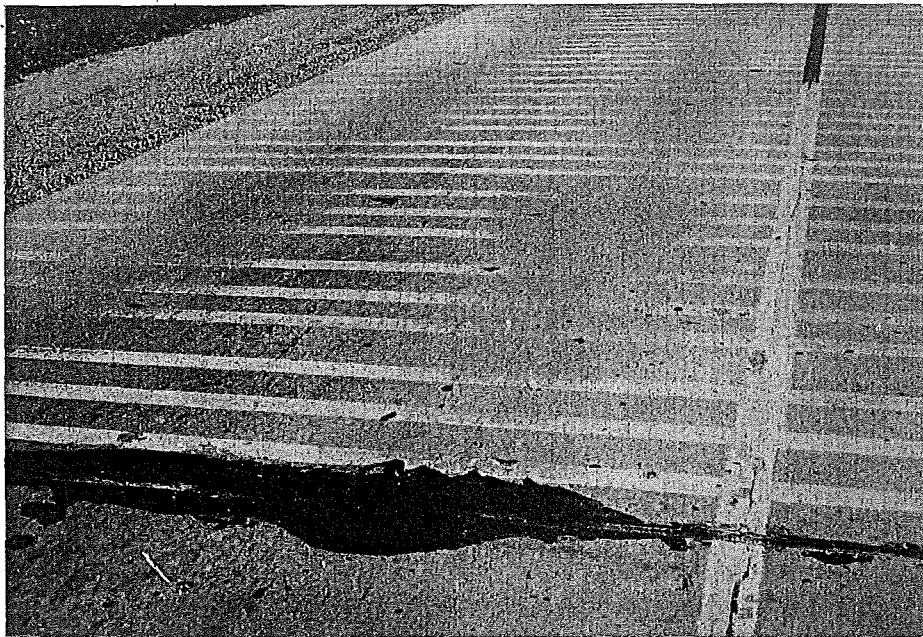
In Test Area 3 (Concrete), paint durability has proved especially low. Traffic density is higher here than in Area 2 (Bituminous).
