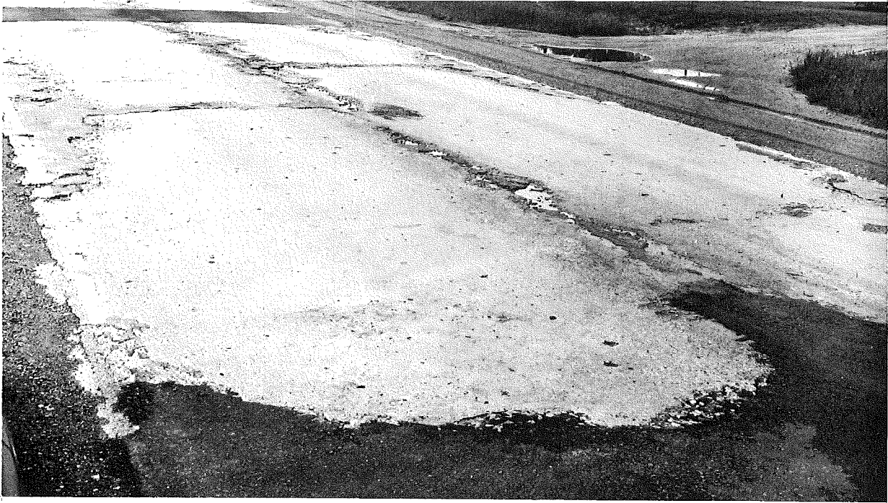
Sta. 227 looking south from the outside shoulder.
