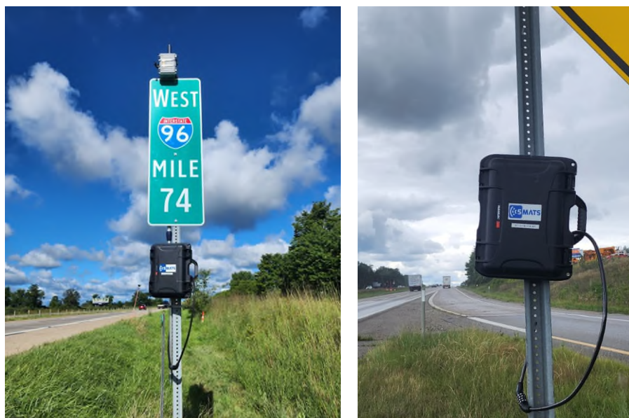
Figure 6-4 Examples of field sensor installation for Bluetooth data collection
