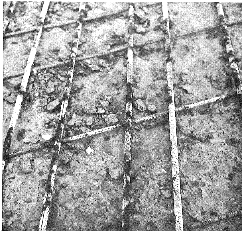
Figure 3. General condition (top) and close-up view of corroded transverse reinforcing bars in 19- by 11-ft area where deteriorated concrete was removed at surface of northbound passing lane.
