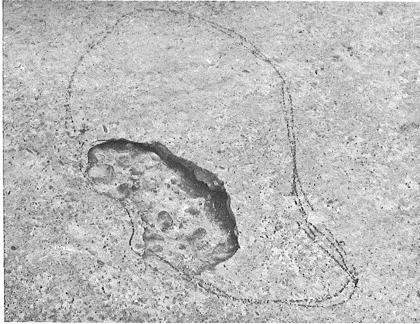
Figure 1. Typical pothole with limits of hollow area outlined in black.
