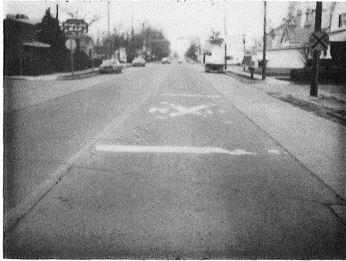
EB M-81 in Reese, Tuscola Co. Approximately 50% of the thermoplastic marking has disappeared. The pavement surface is good.
