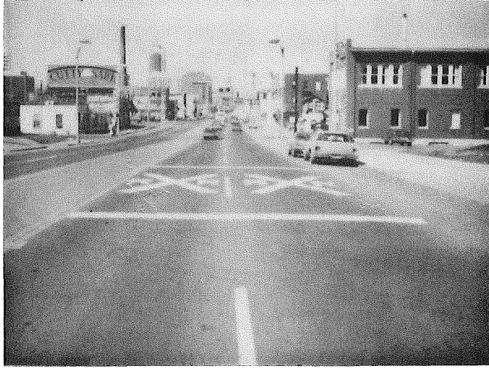
M-143 Michigan Ave. in Lansing The thermoplastic pavement marking is totally intact after one winter.
