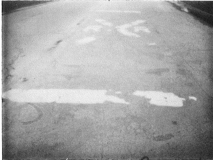
WB M-142 in Pigeon, Huron Co. Approximately 50% of the thermoplastic material remains intact. The pavement surface is not in good condition.
