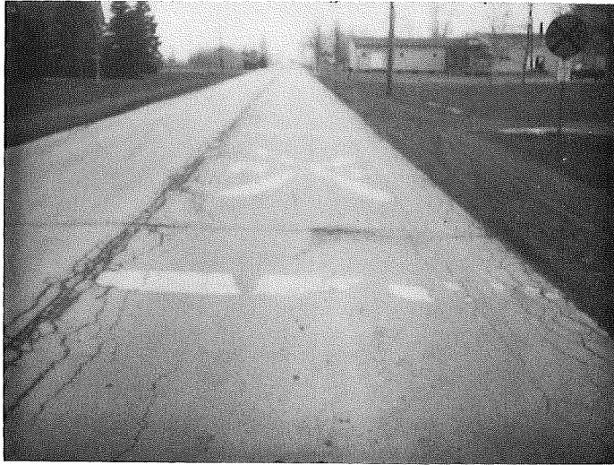
WB M-25 in Unionville, Tuscola Co. Approximately 40% of the thermoplastic marking has disappeared after one winter. Note rough pavement surface.
