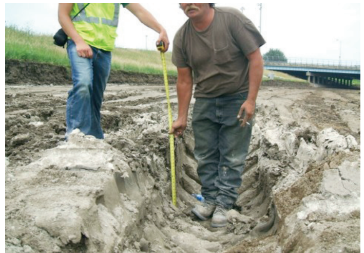
Weak subgrade soils may lead to significant failures under construction traffic loading.
